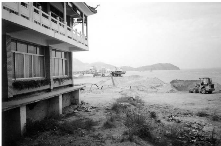
Construction had already begun in Panyu county to develop port facilities for the proposed one-hour access from Guangzhou to Hong Kong.
