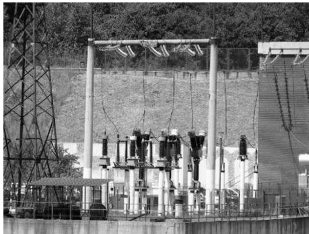
Figure 9.2 An electrical substation.
