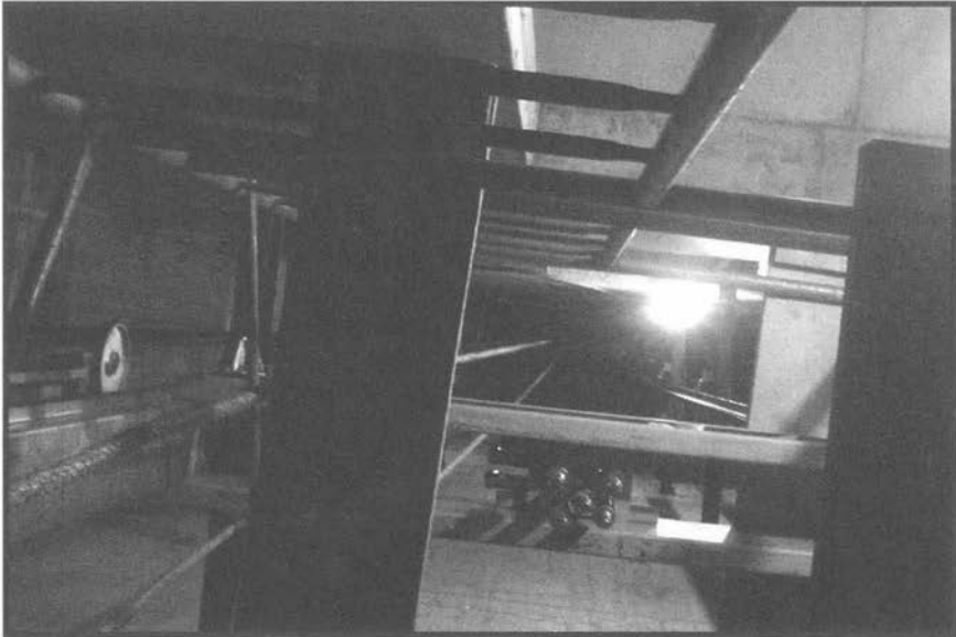
Some elevator shafts, such as this one under construction, provide ladders for easy climbing.
