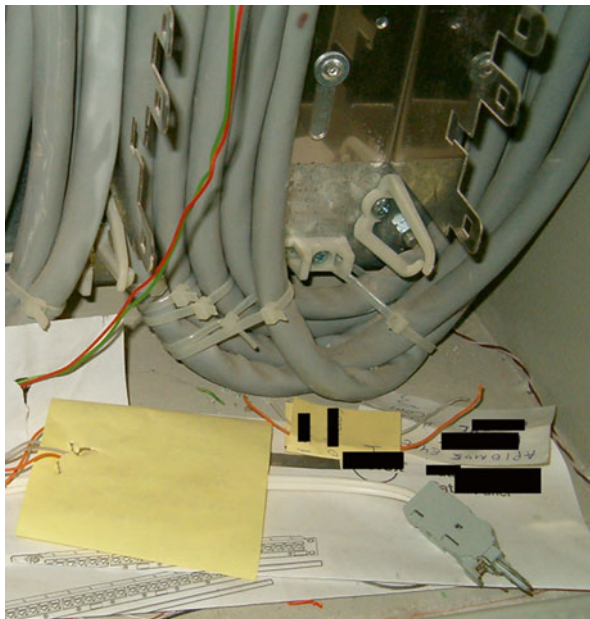
Fig. 4.3 Sensitive information regarding the interconnection of the lines and the tapping tool left at a distribution frame
