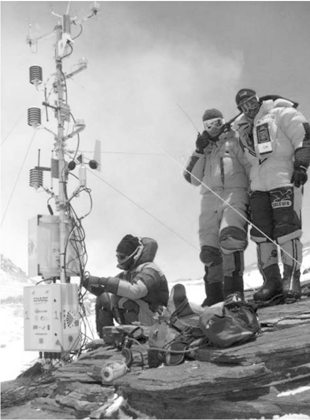
Figure 1.1. Installing the world's highest weather station at 8000 m above sea level on the south col of Mt Everest, May 2011. The summit is 8850 m. Observations are updated hourly on the web – http://share-everest.it/SHAREEverest2011MeteoData/SouthCol/sensorSouthCol.html (Photograph courtesy of the Ev-K2-CNR Committee archive)
