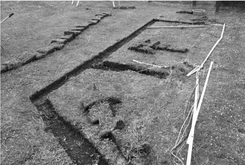
Figure 2.1. Installing a cabled AWS can involve considerable preparation work in digging trenches for cable runs . . . (Photograph by the author)
