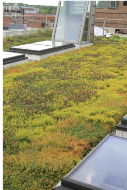
Figure 4.7 Example of a green roof installed by Ann Arbor Architects Collaborative that included rainwater collection for roof irrigation in Michigan. ( Celeste Allen Novak, Architect )
