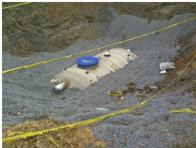
Figure 4.26 Care must be taken during construction to prevent introduction of mud and debris into tank. Note that this inlet pipe is temporarily covered during construction. (Eddie Van Giesen)
