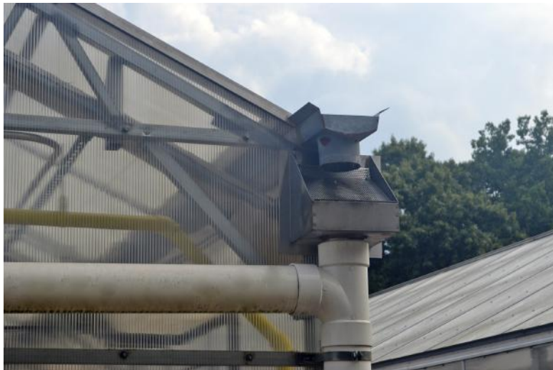
Figure 4.16 This filter has an angled screen, which excludes debris. (Eddie Van Giesen)
