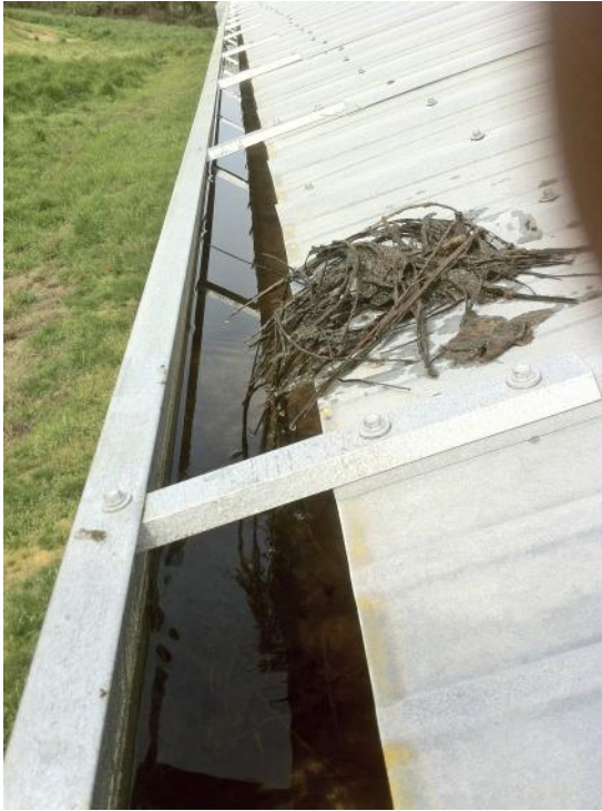
Figure 5.5 Contaminants building up on commercial roof.
