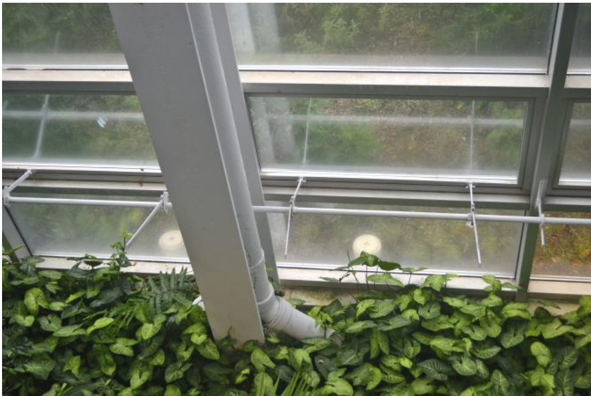
Figure 4.12 Interior downspout attached to conservatory structure recedes into the planting bed on its way to storage. (Eddie Van Giesen)
