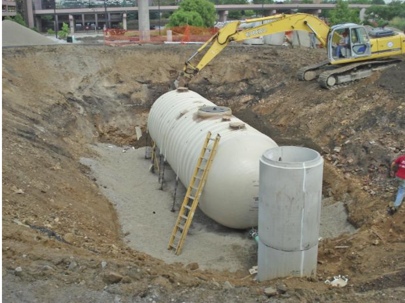
Figure 3.10a Installation of 20,000-gallon cistern for the Metro Intermodal Transit Center in Akron, Ohio, designed by GPD Group. (GPD Group Photo)
