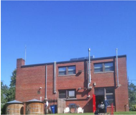
Figure 3.6 The rainwater collection system for Fire Station Number 6 in Raleigh, North Carolina, provides water for toilet flushing. (Celeste Allen Novak, Architect)
