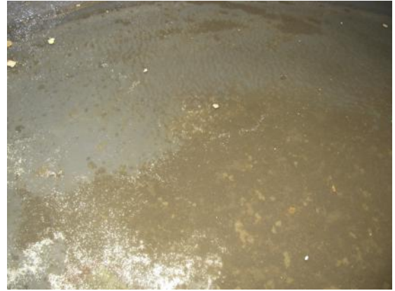
Figure 5.6 Sediments and organic matter accumulate on the bottom of rainwater storage tanks and can become a source of contamination. ( Kathy DeBusk )
