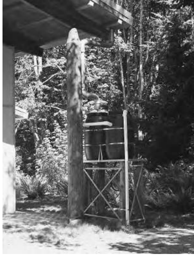
LEFT: Rainwater tanks and roof washer at the side of the building
