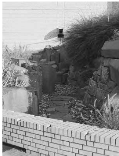
LEFT: Downspout from building to rain garden RIGHT: Downspout to a less-vegetated channel
