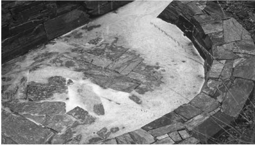
Passive rainwater harvesting: permeable channel below the extended gutters
