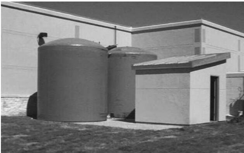
The two 10,000-gallon tanks used for rainwater storage
