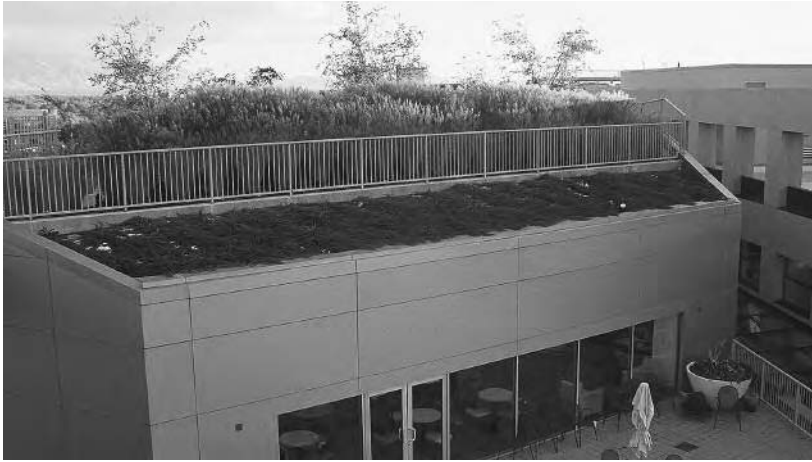
Passive rainwater harvesting: green roof on a library in Salt Lake, UT
