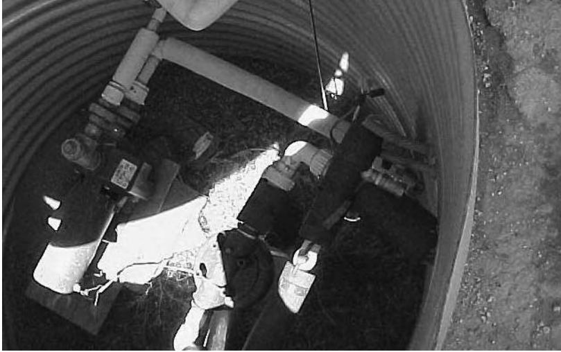
Greywater and rainwater pump and equipment in sump
