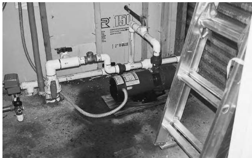
Equipment room with pump and filters
