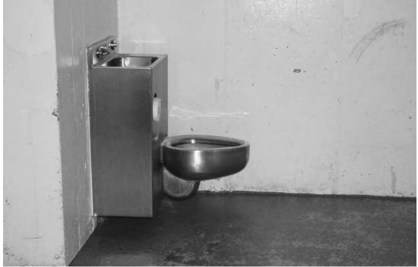
Typical jail toilet
