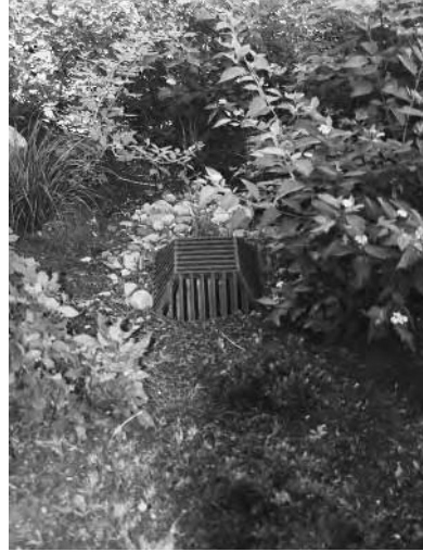
LEFT: Realigned road; note the curvilinear form RIGHT: Drain for overflowing to the next rain garden
