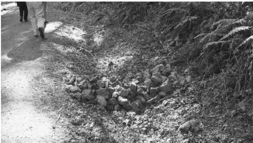
Passive rainwater harvesting: rock weir on a swale
