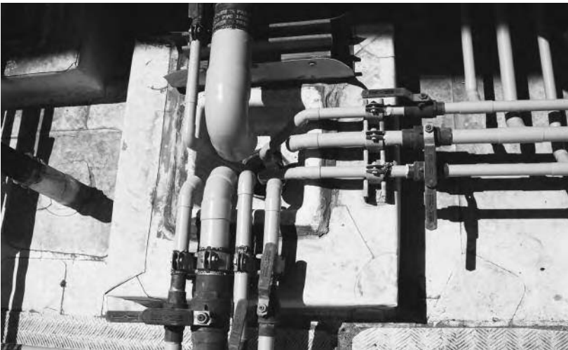
Cooling tower water collection pipe
