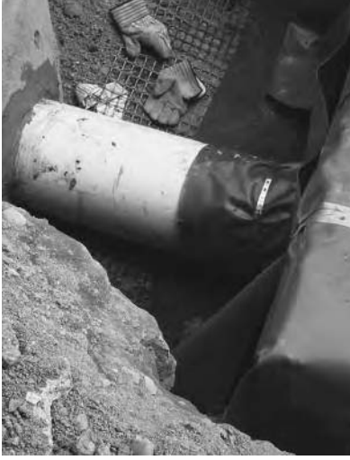
LEFT: Sealing the liner RIGHT: Crates and liner connection to the sump
