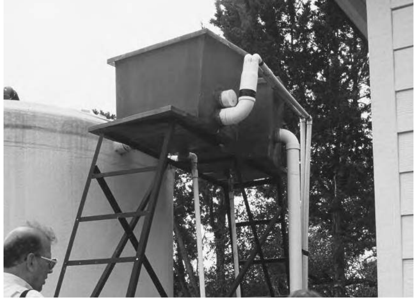
Stay-n-Play Pet Ranch rainwater system roof washer
