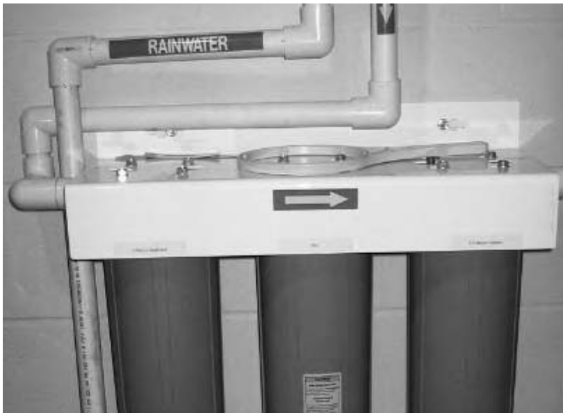
Rainwater filtration system
