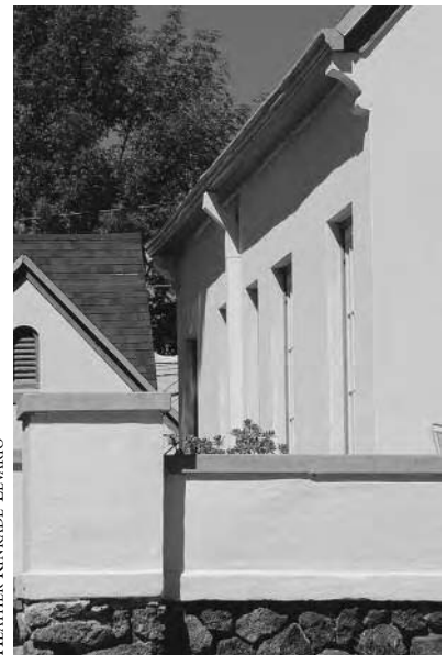
Downspout and gutter on a residential roof
