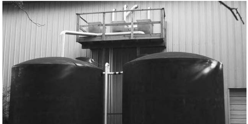
The two cisterns located at the back of the building, with the three roof washers above the tanks
