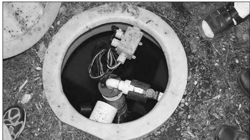
Equipment below-ground access
