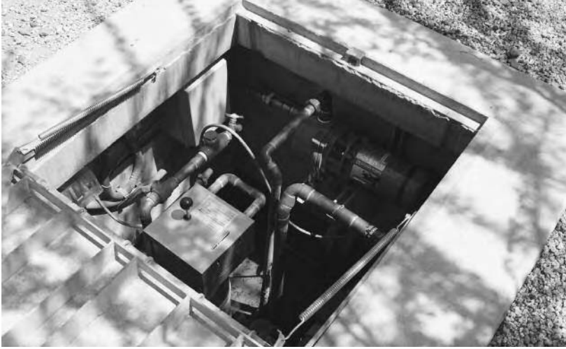
ADEQ equipment vault
