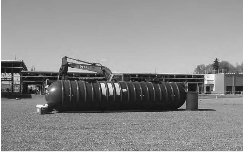
Rainwater 6,000 gallon tank prior to installation
