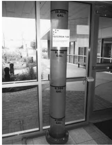
LEFT: Equilibrium tube in the building, used to show the depth of water in the rainwater tank
