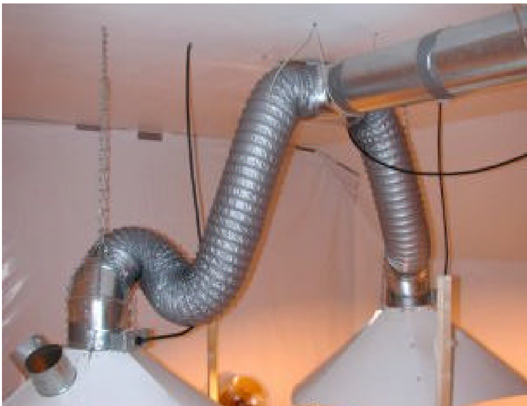
Figure 5.12 - This picture shows two air-cooled hoods attached to their respective air ducts. This photograph is by Chimera.
