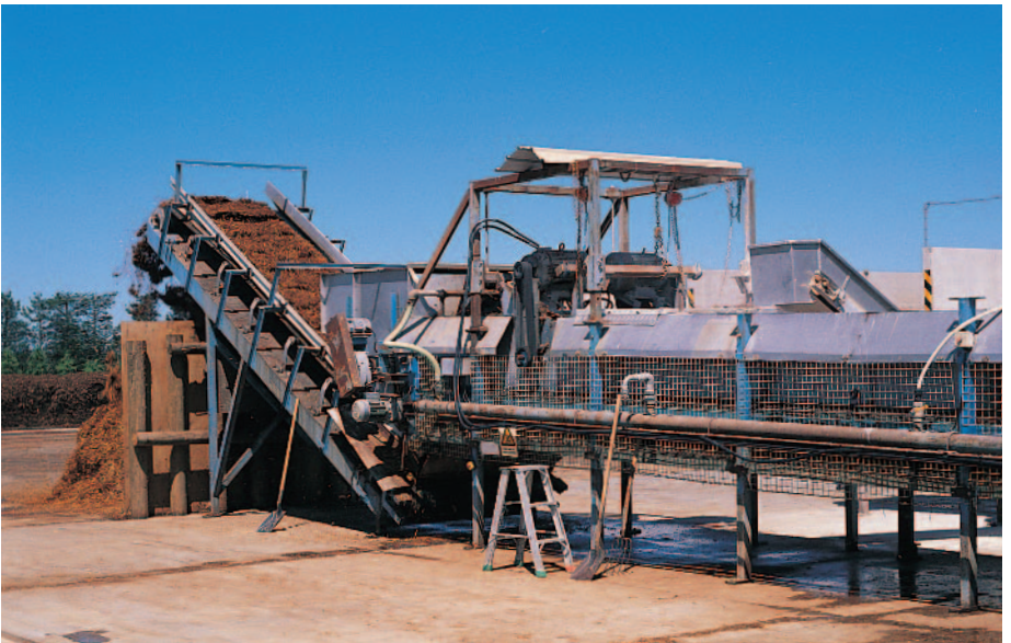
Completion of mechanical assembly. The compost mixture will be placed in piles and ricks (in background) for Phase I composting. Meadow Mushrooms, New Zealand. (Buchanan)
