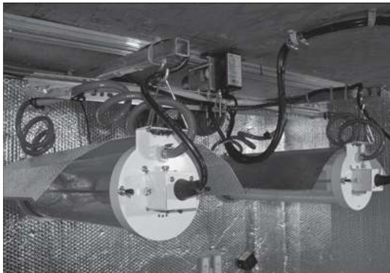
The HID lights in this indoor garden are water-cooled. The waste heat from the lights is used to heat the fish tank.
