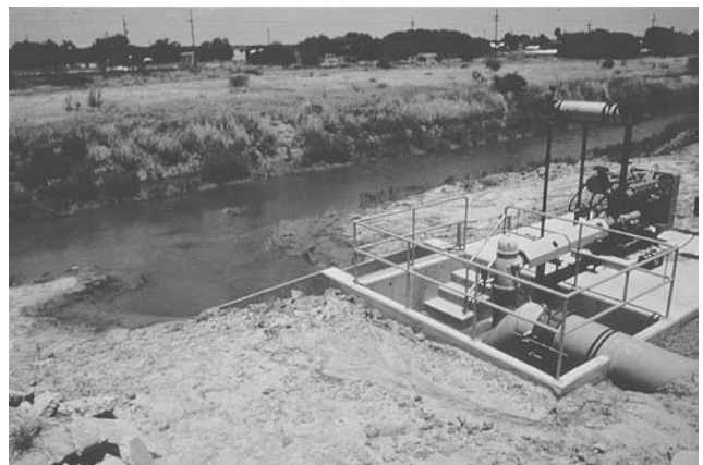
Figure 17. Recirculation water pump at Arroyo Aquaculture Association farm in Texas. (Photo by Louis Hamper.)
