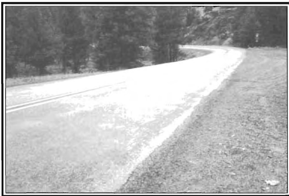
The overspray on the gravel at the edge of the lane is a clue that the surface is coated with slippery oil.
