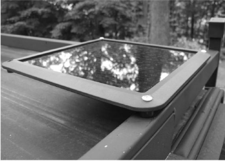
Solar battery trickle charger mounted to exterior of BOV
