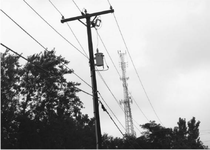
Communications tower vulnerable to disaster
