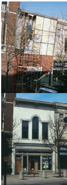
Demonstration project Before and after of a shop used as a neighbourhood planning office and as a demonstration for improving street frontages.
