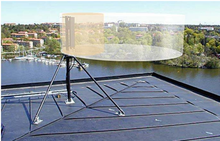
Figure 3. Compliance boundary: Roof-mounted 3G (WCDMA, 2,100 MHz) antenna cylindrical compliance boundary (for ICNIRP occupational and general public limits) diameter: 3 m, height: antenna height+20 cm (courtesy of C Törnevik, Ericsson Systems, Sweden).
