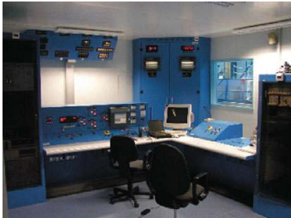
Figure 25 MINERVE reactor control room
