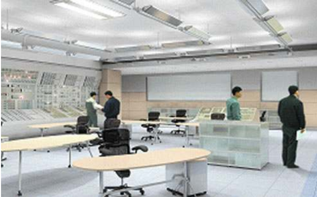
■ Figure 6 Main control room (Courtesy of Korea Hydro and Nuclear Power Co., Ltd.)
