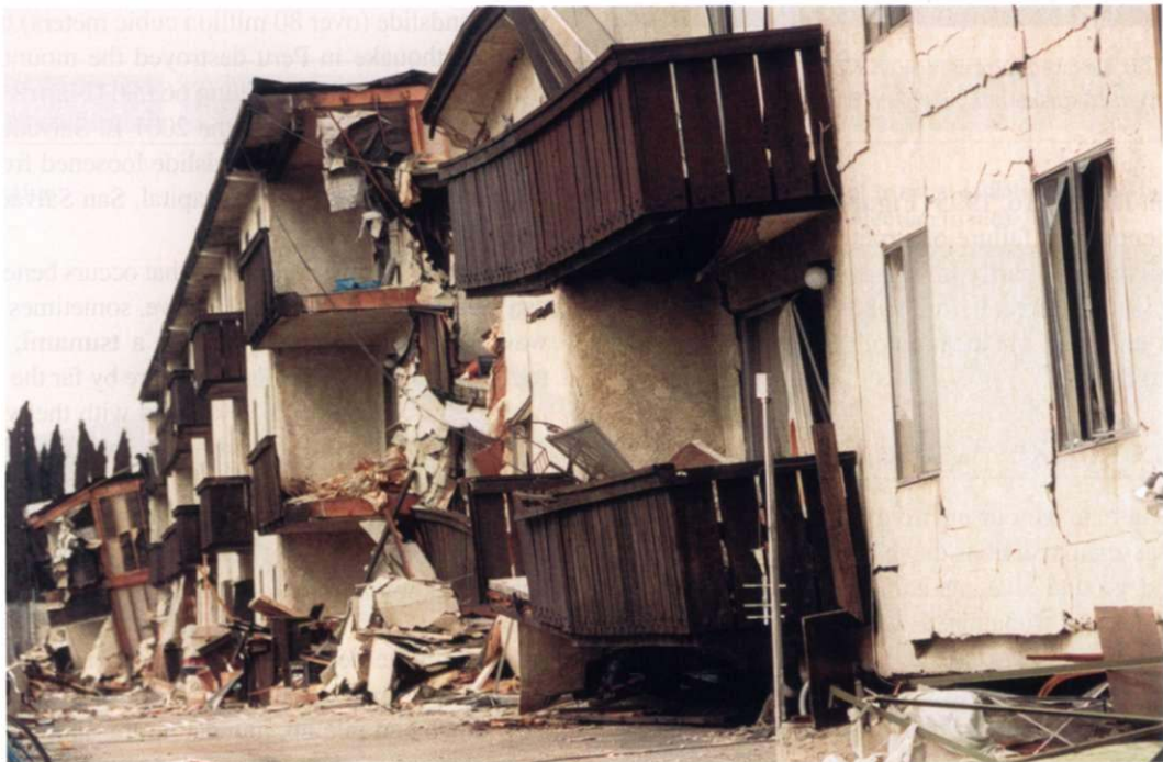
Figure 13.14 Sixteen people died in the Northridge Meadows apartment building in Los Angeles during the 1994 Northridge earthquake. The victims lived on the first floor and were crushed when the upper levels collapsed. Many more buildings would have
