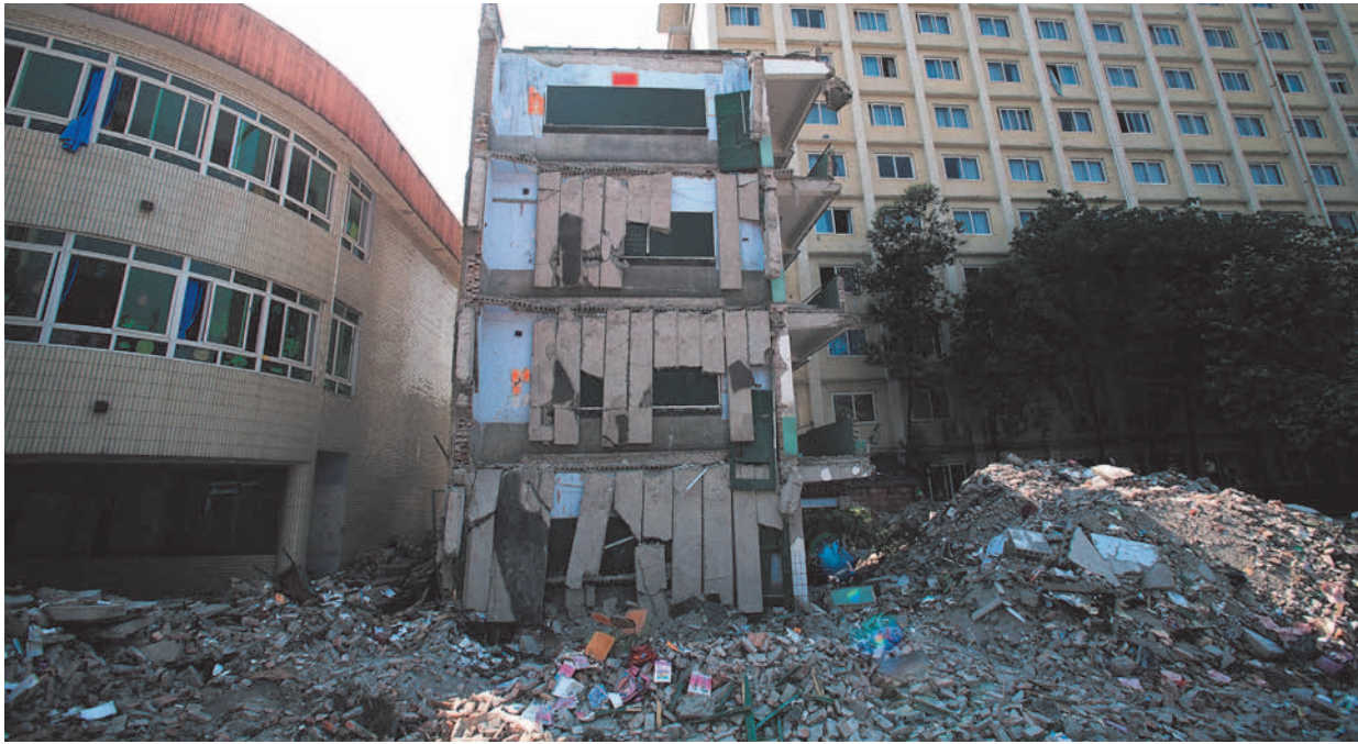
FIGURE 6.7 Earthquake damage and building standards
