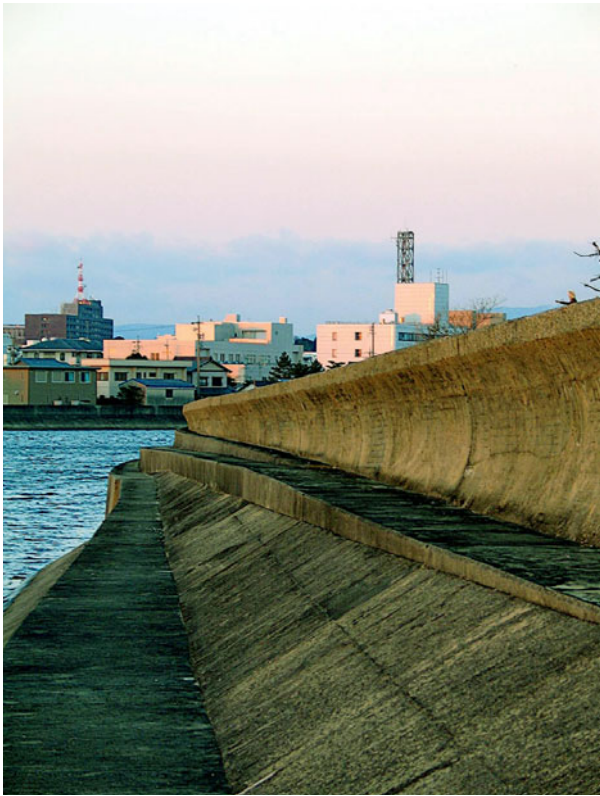
Fig. 8.22 A 16 m high massive concrete wall against tsunami impact at Tsu-shi, Japan. (Photo credit: Chris O at en.wikipedia)
