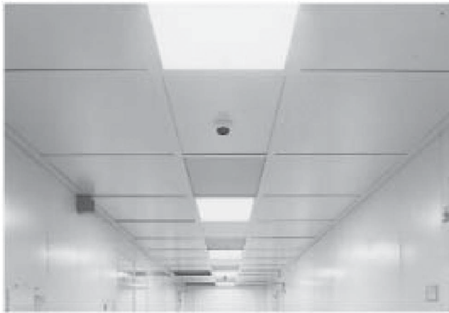
FIGURE 9 A suspended ceiling utilizing lay-in panels and lay-in lighting troffers. A variety of cleanable materials can be used for the panels. The lay-in lights should be of a design that will provide appropriate service based on the cleaning protocol to be used. (Courtesy of CleanTek.)
