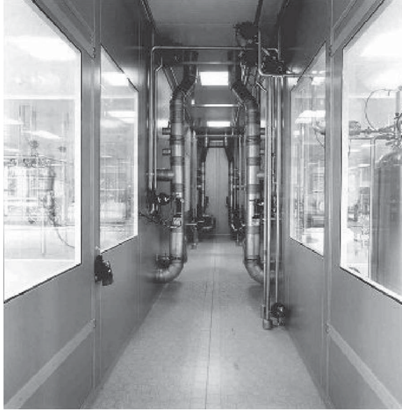
FIGURE 19 The utility chase is located between two clean rooms. Major utility lines are installed within the chase and hook-up lines for local pieces of process equipment are connected through the clean-room walls. A major benefit of this arrangement is that installers need not be fully garbed in clean-room attire to access the utility lines. (Courtesy of CleanTek.)
