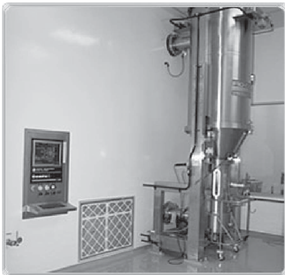
FIGURE 8 A modular wall system has been installed in a manner that provides a smooth surface for cleaning. The fit of the components and the method of sealing are important when a modular wall is selected. (Courtesy of Portafab.)
