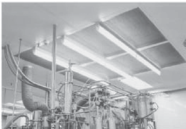
FIGURE 10 An area of HEPA filters is installed above a process machining. Tear drop lighting is used to permit maximum filter coverage. A monolithic ceiling construction of gypsum panels suspended from a framework. The panels are finished with an epoxy coating compatible with cleaning/sterilization procedures. (Courtesy of CleanTek.)
