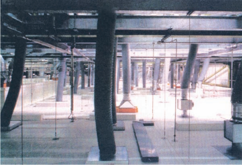
Figure 16.13 Walkable ceiling interstitial space. The air handling units are on the grating floor above. The walkable ceiling allows easy access to HVAC control instruments and dampers, as well as allowing for the servicing of lights from outside the clean envelope. (Courtesy Clestra Cleanrooms Inc.)
