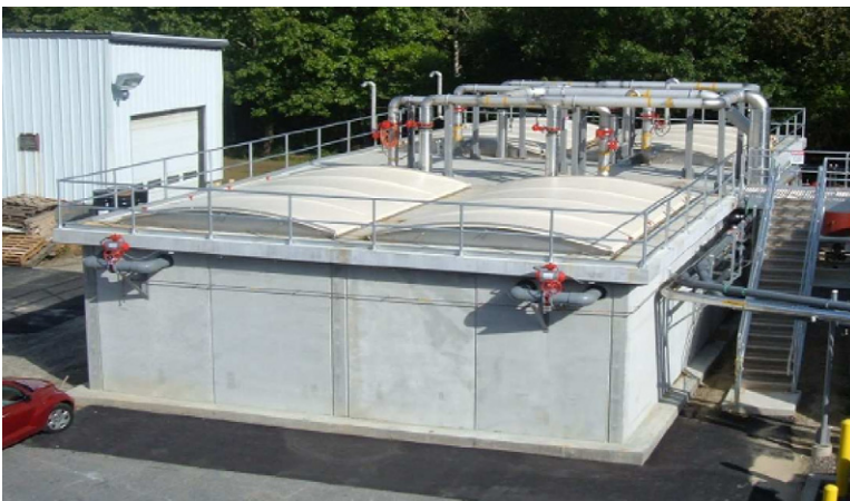
FIG. 5.13 The covered aniMBR tanks at Ken's Foods.
