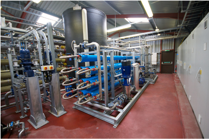
FIG. 5.53 The RO skid at Kanes Foods.
