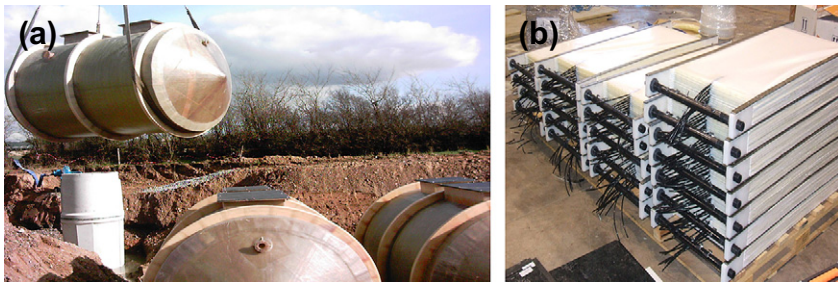
FIG. 5.16 (a) Installation of the tanks at Feenagh and (b) the membrane modules.
