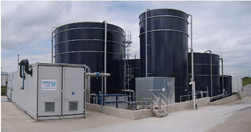
FIG. 5.54 The Dairy Crest plant at Foston.
