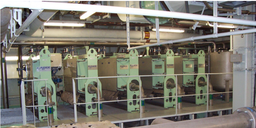
FIG. 5.57 Pleiade ® skid on the Queen Mary II.
