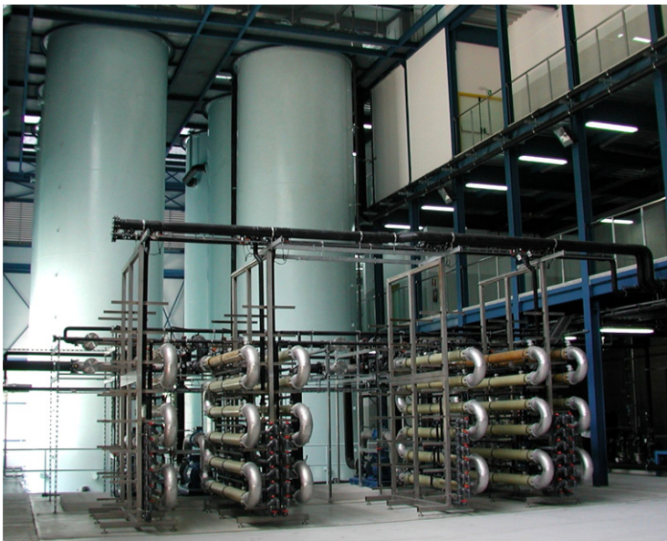
FIG. 5.50 The Wehrle sMBR landfill leachate plant at Bilbao showing the tall bioreactor towers and sidestream membranes.
