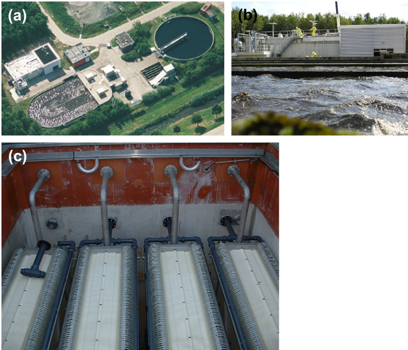
FIG. 5.21 Heenvliet WwTW: (a) from the air, (b) from the side and (c) inside the membrane tanks.
