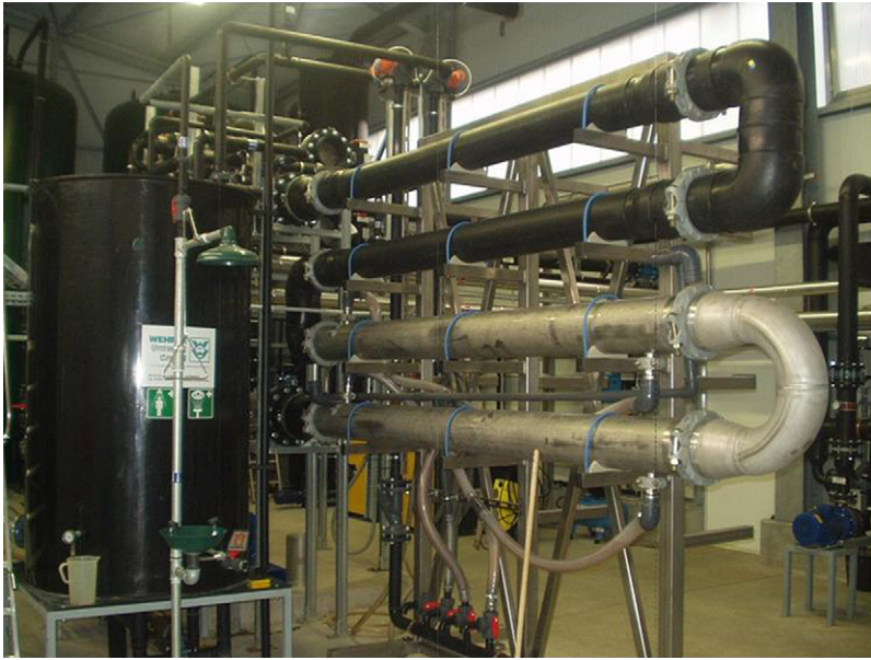
FIG. 2.23 sMBR pilot plant: the total retentate fluid path is four times the length of one horizontal module.
