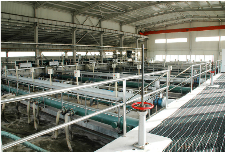
FIG. 5.49 The membrane tanks at Miyun.
