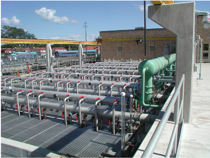
FIG. 5.35 The MBR at Traverse City WwTW, showing the permeate and air headers.
