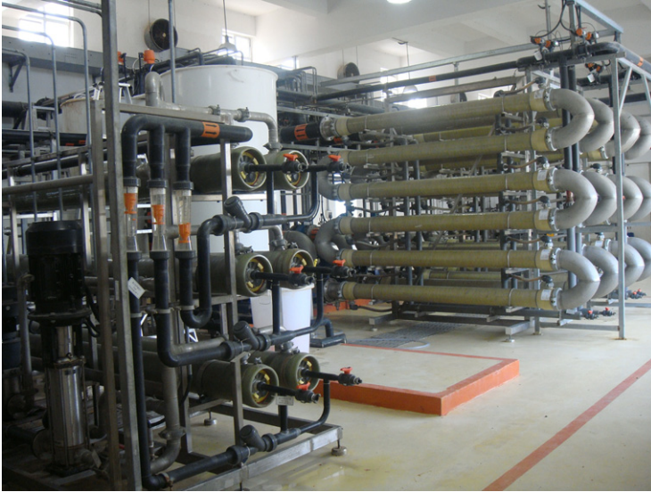
FIG. 5.55 The membrane skids at Baishi Ao, Foshan City: NF (left) and UF (right).
