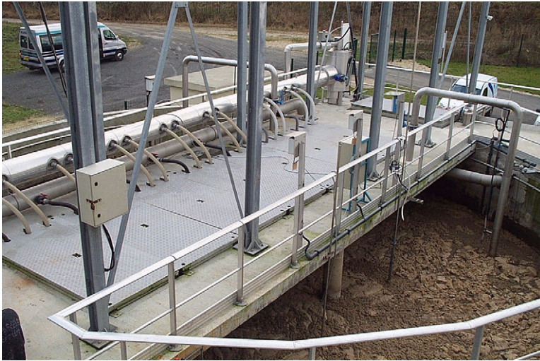
FIG. 5.27 Aeration tank and covers, Perthes en Gatinais plant.
