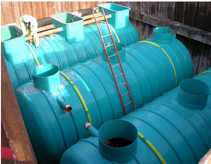
FIG. 5.24 The storage and biotreatment tanks at Selborne, UK.
