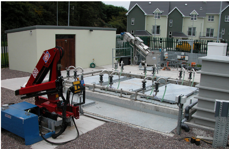
FIG. 5.15 The plant at Halfway. The screen is located mid/top picture, with the inlet pump chamber behind it. The anoxic tank is below the screen, and the MBR is the covered tank with the swan-neck air feed lines. The sludge tank is located behind the MBR and to the right of the anoxic tank. The permeate pump chamber is behind the sludge tank.
