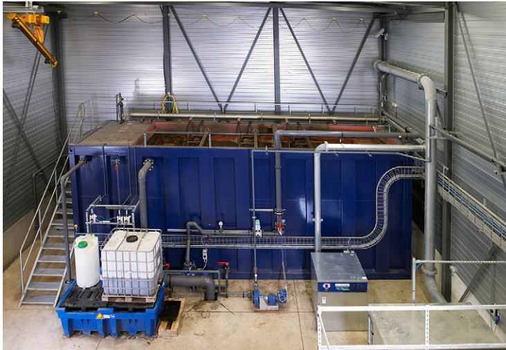
FIG. 5.25 The MBR installation at Oerlemans.
