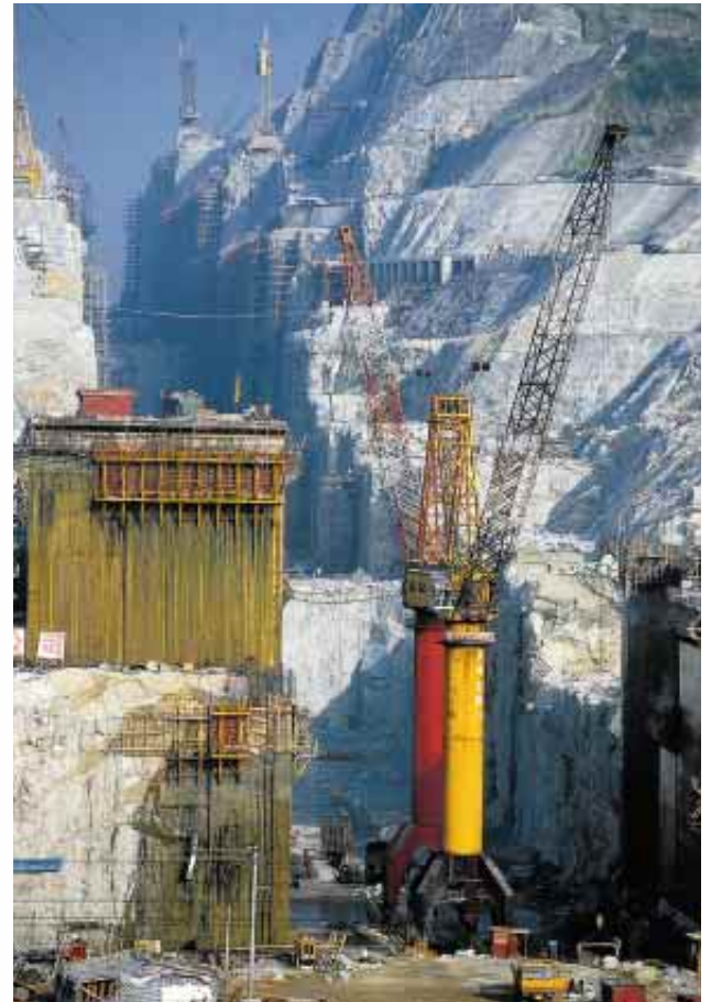
GIGANTIC LOCK: Matching the dam in scale, an enormous five-step lock ( right ) is being carved from granite on the river's left bank. The chambers of the lock will be lined with concrete, and when completed it will lift 3,300-ton ships 285 feet, making it the largest such system in the world.
