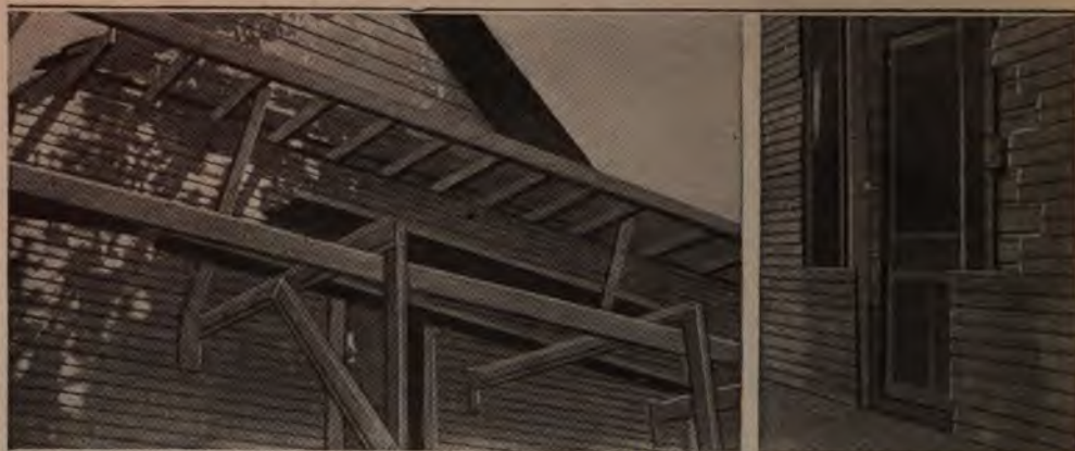
PHOTO COURTESY GEDNER HOOVER The Side View Shows the Narrow Weather Boards of the New Structure being Built a Few Inches Away from the Old One. The View of the Front Door Also Indicates the Small Space between the Two Walls, and the Necessity of Having the New Doors Correspond in Position to the Old Ones
