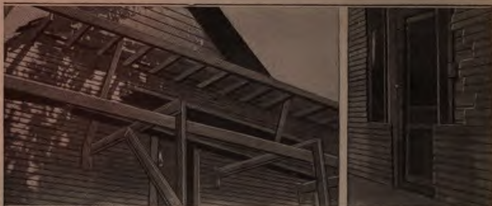
PHOTO COURTESY BISHOP MOVIER The Side View Shows the Narrow Weather Boards of the New Structure being Built a Few Inches Away from the Old One. The View of the Front Door Also Indicates the Small Space between the Two Walls, and the Necessity of Having the New Doors Correspond in Position to the Old Ones
