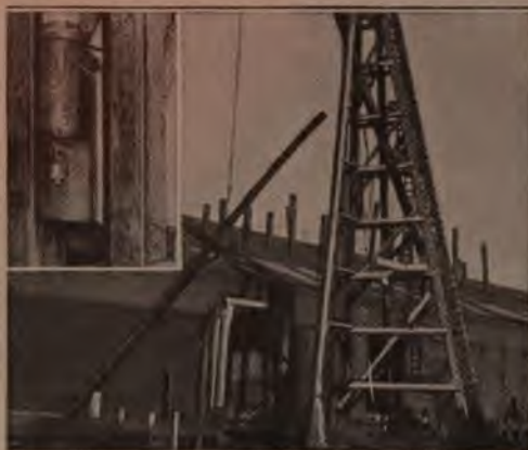
When the Boom is Not in Use, It is Tied Fast to the Pile Driver, in Such a Manner That It Does Not Interfere with the Operation of the Hammer
