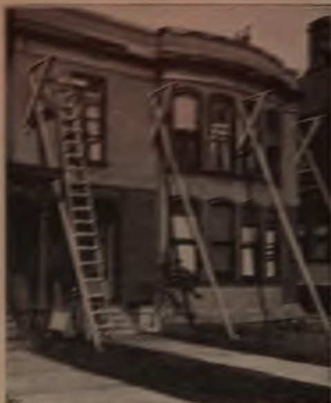
Brackets for Scaffolding Supported by Long Braces Reaching to the Ground are Found Useful on Repair Jobs
