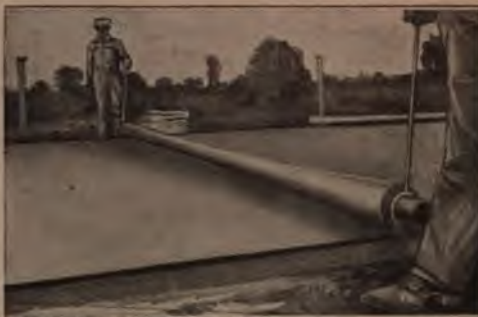
The Roller Tapers to a Smaller Diameter near the Middle, and Thus Automatically Rolls a Concrete Road to the Correct Pitch for Drainage
