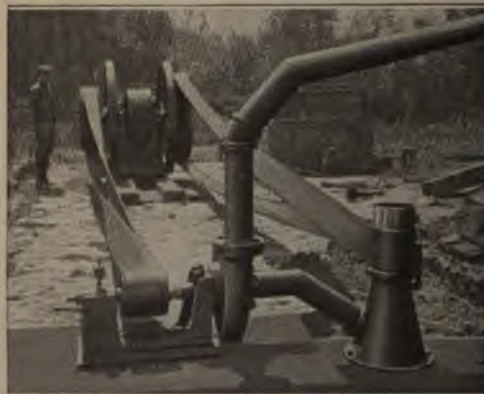
The Screw Pump Raises the Water to the Surface, and the Centrifugal Pump Then Takes Hold and Throws it Up to the Storage Tank
