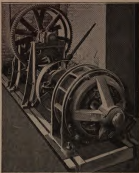
A Substantial Foundation for Motors and Machinery Which Permits of Easy Adjustment or Removal of the Machines
