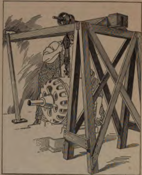
This Support for Differential Tackle was Devised in an Emergency for Taking Down a Generator
