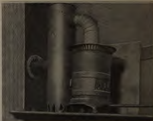
This Heating Arrangement Overcame Troublesome Freezing of Water Pipes in Cold Weather, and was Cheaply Installed
