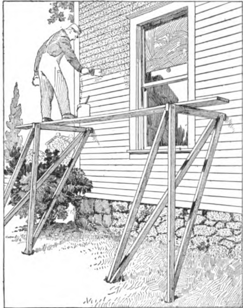
These Supports for a Scaffold Are More Convenient than the Use of a Ladder, Especially for Work at a Comparatively Low Height
