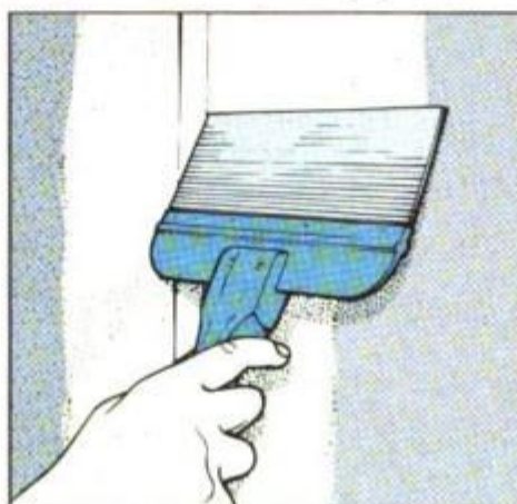
19 Once both sides of the tape are embedded in the joint, add another coat of compound to one side using an 8-in. knife.
