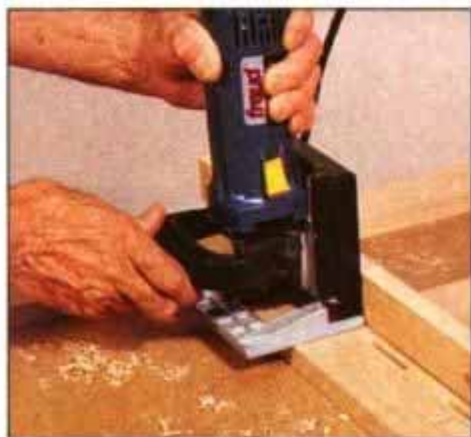
3 After marking for frame-to-case plates, lay frame on bench to cut slots. Use guide strip to locate divider-stile slots.
