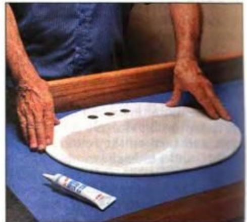
20 Apply a bead of caulk around the cutout before installing sink. Also apply caulk under oak backsplash before securing.
