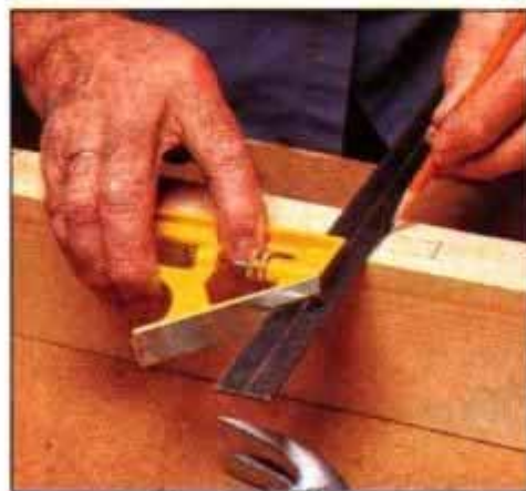
7 With the beam halves nailed together temporarily, use a square to lay out the wedge mortises on the beam edges.
