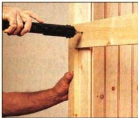
6 After back frames have been assembled, secure the beaded paneling with glue and screws driven from the back of frame.
