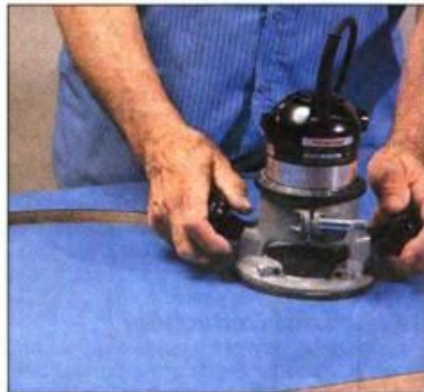
19 After the laminate has been glued to the top, bore a starter hole and rout the cutout with a flush-trimming bit.
