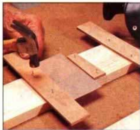
8 With plywood mortise template tacked in place, use a cardboard spacer to position router guide strips on one beam half.
