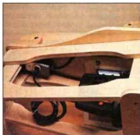
18 After attaching the outlet box, single receptacle and switch to the base, connect switch and receptacle with 16/3 wire.
