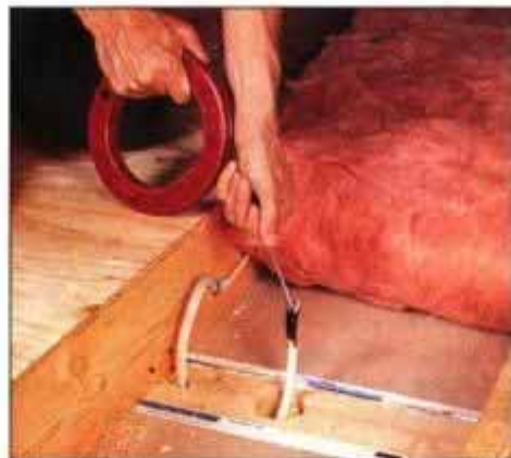
6 From the attic, carefully pull up the fish tape and the new cable through the wall and over to the ceiling fixture box.
