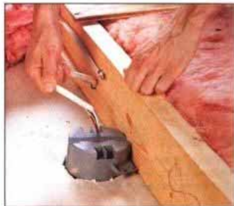
7 Feed the new 3-wire cable into the ceiling box. Cut the cable to length and strip 10 in. of sheathing from the ends.
