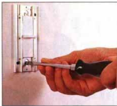
10 Tuck all the wires into the box and secure the dimmer switch. Tighten the two screws until the switch feels snug.
