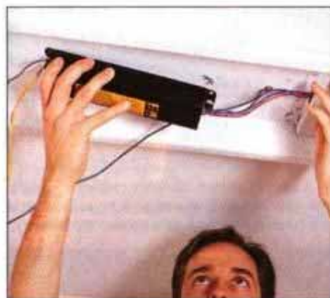
13 Remove the old fluorescent ballast by loosening the screws or bolts that secure it to the metal fixture channel.
