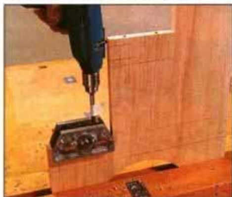
6 Before attaching the rails to the sides, mark dowel locations on the steps and then bore on these marks.
