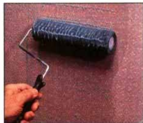
2 Use the porous roller to apply a thick layer of remover. Then, allow the gel to set for approximately 15 to 20 minutes.
