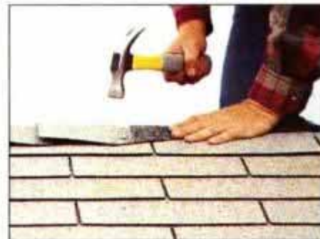
14 Cut the shingles into three tab-size pieces and use the tabs to cap the peak. Be sure to space each piece 5 in. apart.
