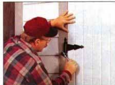
16 Hang the door with three steel gate hinges. Secure it to the trim with lagbolts, then add the handle, bolt and hasp.
