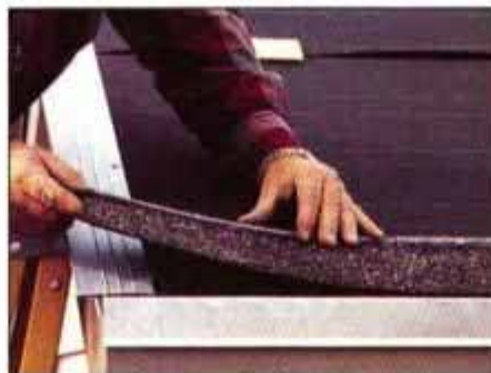
13 After nailing the drip edges in place, trim the tabs from the shingles and then install a starter row along the eaves.
