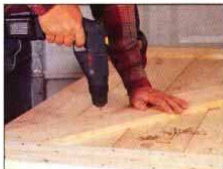
15 Build the door by using tongue-and-groove pine. Attach the crossmembers and a diagonal brace with screws.
