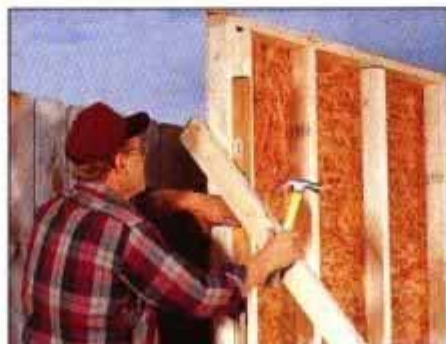
5 Set the first wall up and nail it through the soleplate. Then, level and brace the wall with a 2 × 4 nailed to the floor.
