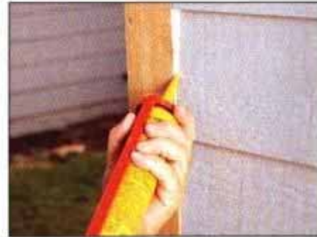
12 Caulk all siding-to-trim joints and soffit joints. Always apply sparingly and avoid smoothing it with a finger.
