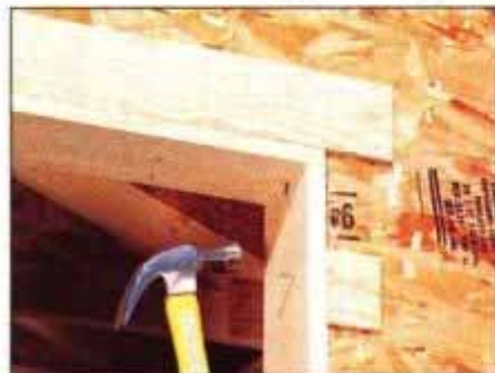
10 Use 1 x 5 pine for the doorjamb. Align with 1/4-in. plywood face-trim shims. Place shims under the corner trim as well.
