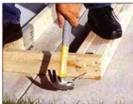
3 Nail each stud through the plates with two 16d nails per stud. Place triple studs at the ends of both long walls.
