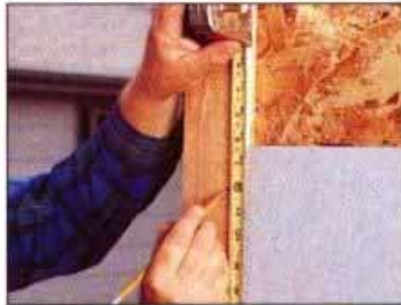
11 To keep the siding lapped uniformly, measure up from starter row and mark the spacing on the trim in 6-in. increments.
