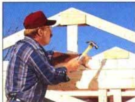
8 Lay the trusses between the walls and then tip up the end trusses. Center and toenail them to the wall top plates.
