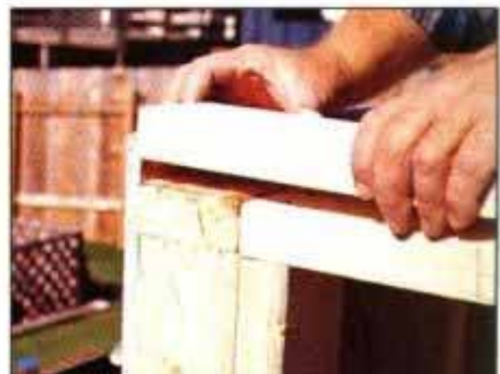
6 After the end walls are set up, add a second top wall plate. Overlap the wall plates at the corners and nail in place.
