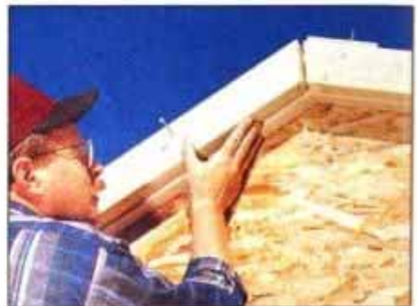
9 Create a 3-in. roof overhang at the gable ends by adding double 2 × 4 rafters to the truss rafters already in place.
