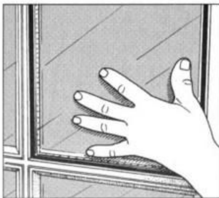
19 Press the new pane into the sash. Apply even pressure to seat it firmly and allow excess silicone to squeeze out.
