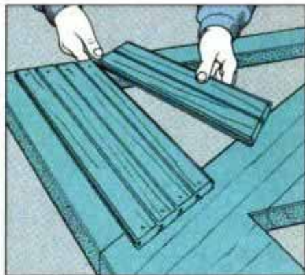
12 Install 5/8-in.-thick beaded fir to the inside surface of the stringer assemblies. Nail in place with 4d galvanized nails.
