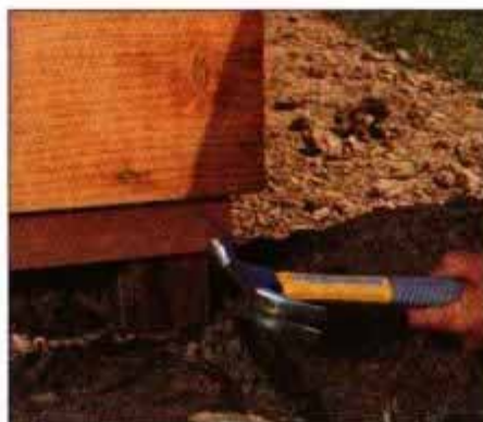
17 To conceal the exposed truss plates on the posts, install a skirt of 1 × 3 redwood. Rip it from 1 × 8 stock.
