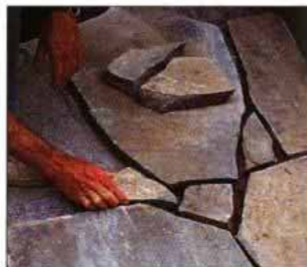
12 Lay all the large stones in place first, then fill in the gaps with smaller stones. Gaps should be 1 in. wide or less.
