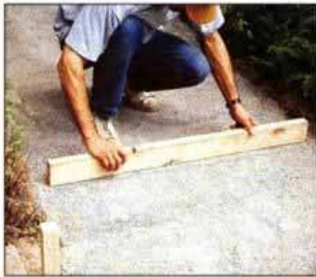
5 Use a 2 × 4 screed to even out the crushed stone. A uniform base at this point provides a useful reference for later work.
