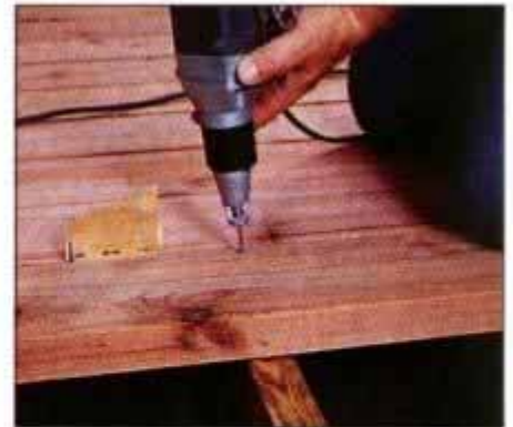
9 Use a 1/4-in. plywood spacer to maintain consistent gaps between planks. Drive two screws through each board into each joist.
