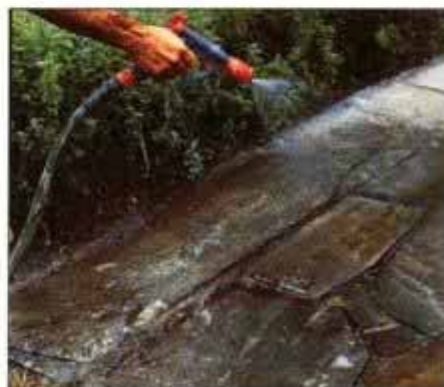
15 Finish up by giving the walk a thorough rinsing. This will remove the stone dust and further compact the joints.
