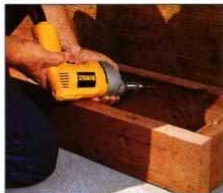
18 Build a step box from 2 × 6 material and screw it to the deck face. Bore oversized screwholes to allow for movement.
