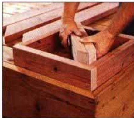
11 Build the square corner boxes, then install two mitered crosspieces in each to support the mitered seat planks.
