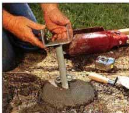
1 After pouring each footing hole, set a 4 × 4 bracket into the wet concrete. Align the brackets with the string line.
