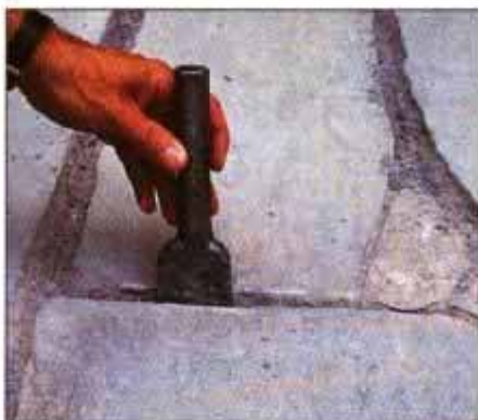
14 To keep the large stones from shifting, use a wide-blade mason's chisel to pack the joints as tightly as possible.
