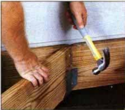
7 Use 45° joist hangers to attach the joists to the angled ledger. Nail the top half of the joist directly into the ledger.
