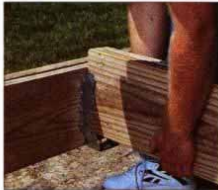
8 Double joists require double-wide hangers. Install these hangers on the rim joist, then slide the two joists into place.
