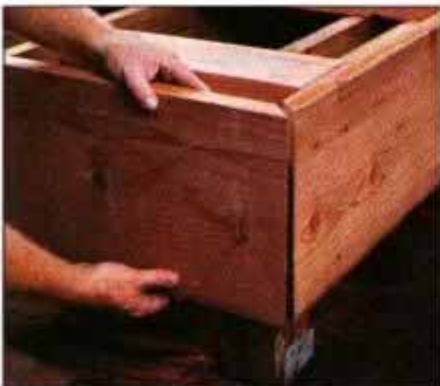
10 Trim the perimeter of the deck with 2 × 12 redwood. Screw these boards into the rim joists and also into the deck planks.
