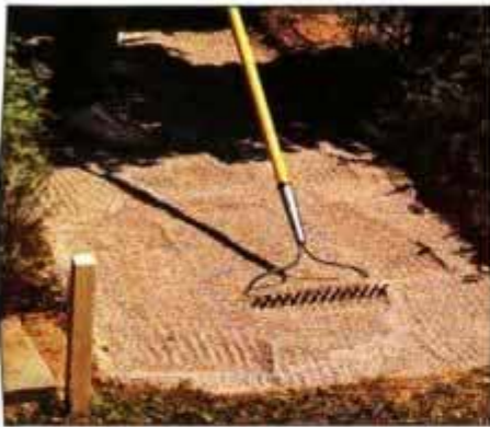
4 Spread crushed stone over the fabric to a depth of about 4 in. Make sure all the corners are filled, then rake the surface flat.
