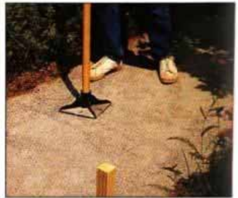
6 Once the bed is basically flat, use a hand tamper to compact the crushed stone. Compact the area uniformly.
