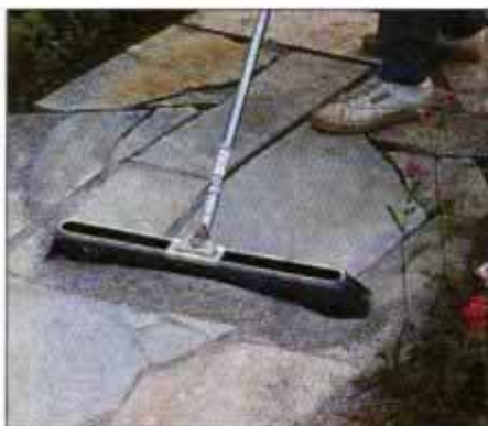
13 When you're finished laying the flagstone, spread crushed stone over the surface and into the cracks with a broom.
