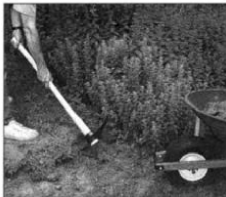
2 Using a pick and shovel, remove all the sod, stones and other obstructions to a depth of about 4 in. Rake the bottom flat.
