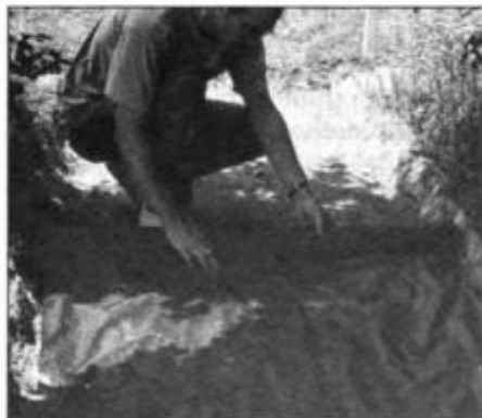
3 Tamp the soil in the work area and then cover the excavation with landscape fabric. The fabric inhibits weed growth.
