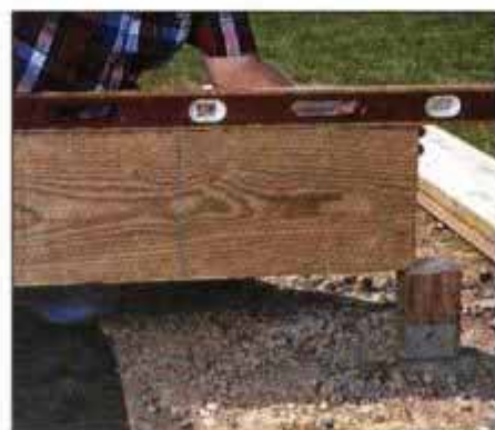
5 Use a straight joist to level between the ledger and the support posts. Mark and cut the posts, then check the level again.
