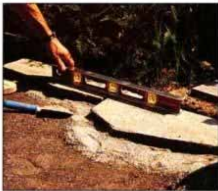
8 Level each ensuing stone in place. Because the surfaces are rough, the level is bound to rock. Shoot for approximate level.
