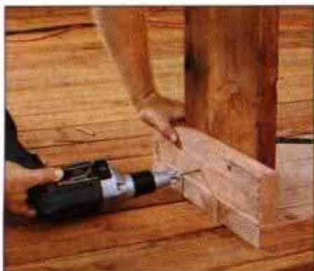
13 To make the bench legs, cut 14½-in.-long pieces from 2 × 12 stock and center them on the crossmembers. Screw in place.
