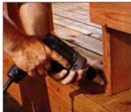
15 Bore the clearance holes diagonally through the bench legs and into the decking. Then drive screws into the holes.
