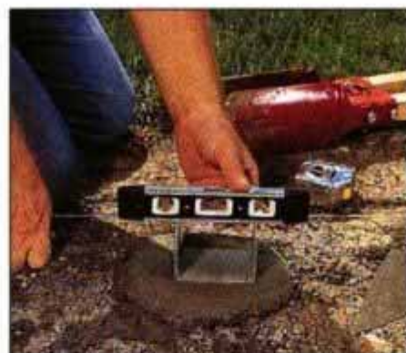
2 Level the 4 × 4 brackets in both directions using a torpedo level, and let the concrete set a day before building on it.
