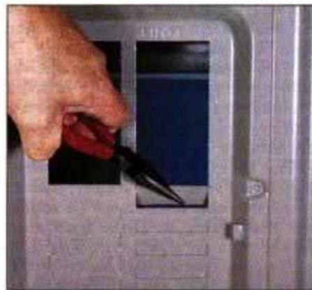
19 Use pliers to twist a breaker-slot plate from the panel cover. Then, replace the cover and energize the panel.
