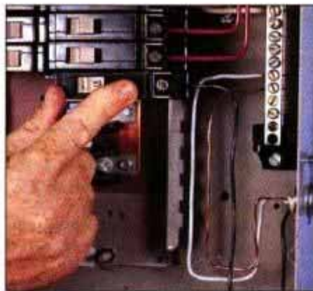
18 Secure the black, hot wire under the lug of a 15-amp breaker. Then press the breaker onto its hot-bus prong.
