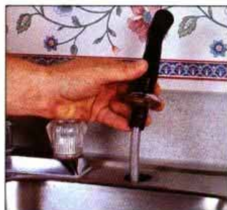
9 Disconnect the old spray hose at the faucet port. Then, loosen the spray hose jamb nut and lift out hose and deck fitting.
