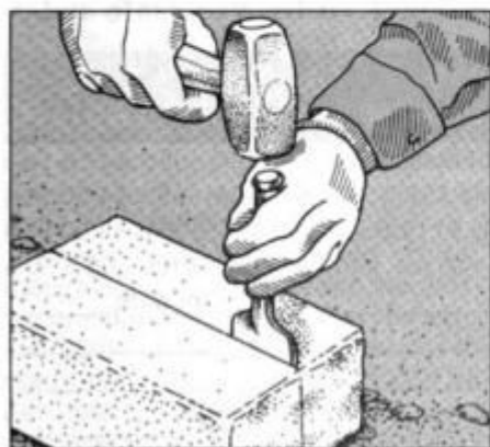
17 Using a mechanics hammer and mason's chisel, score all the cutlines. Then break the block in half with a single blow.
