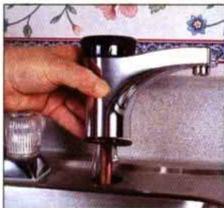
11 Straighten the supply tubes attached to the heater faucet and insert through the sink's deck hole from above.
