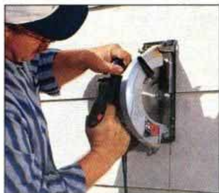
9 Using the holes as a guide, mark the opening and cut through the siding and sheathing with a circular saw.
