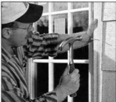
14 Temporarily secure the door by driving 12d galvanized casing nails through the molding. Leave 1/2 in. of nail showing.
