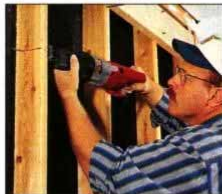
4 Cut studs at header location. Use a circular saw to start the cuts, then finish the job with a reciprocating saw or handsaw.
