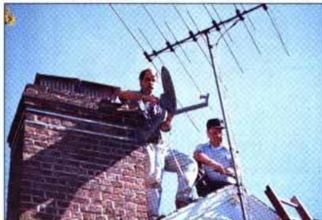
New antenna for old: For chimney mount, Scherer (left) and Akers preferred stainless-steel to galvanized straps.
