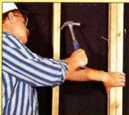
1 Use an existing stud as the first king stud. Nail a jack stud to this stud and then toenail it to the soleplate.
