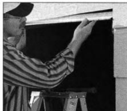
13 To protect the header and door casing from rot, install a sheetmetal rain cap under the top section of the siding.
