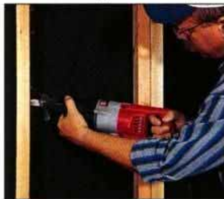
5 Use a reciprocating saw with a metal-cutting blade to cut the nails that hold the sheathing and siding to the studs.
