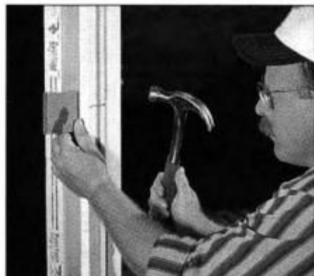
15 After checking door alignment and operation, shim casing and drive 8d casing nails through casing, shims and jack studs.
