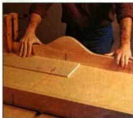
12 After planing the panel stock to 3/8 in. thick, use a crosscut table mounted on the table saw to make square panel cuts.
