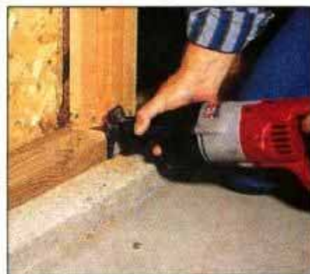
10 Where the circular saw can't reach, use a reciprocating saw from the inside. Cut through the soleplate, as well.
