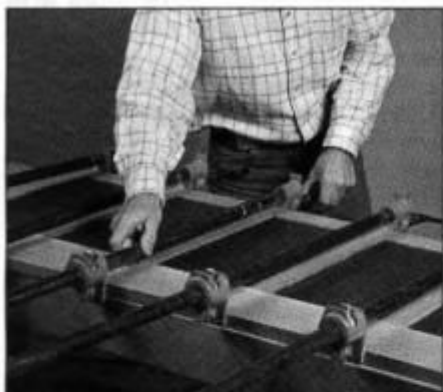
15 Apply glue to the stile tenons and to the rail grooves at the stile locations. Panels are held in grooves without glue.
