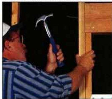
6 Lift the header into place and secure it to the king studs by nailing with 16d nails. Use four nails per header end.
