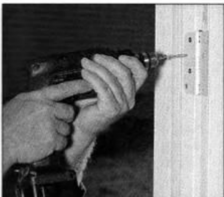
16 Fill open holes in hinges with long screws. Drive these screws through the casing and into the jack stud.
