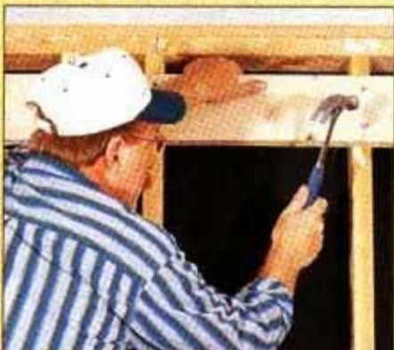
2 After the second king and jack studs are in place, support the wall by nailing an 8-ft. 2 x 6 across the studs near the ceiling.
