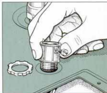
22 Slide the threaded end of a conduit connector into the knockout hole and tighten it in place with the connector nut.
