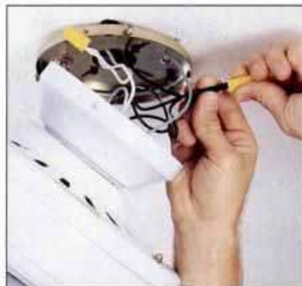
11 Hang the assembly from the mounting plate using a wire hook. Then, attach like-colored wires with wire connectors.
