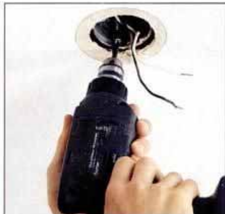
5 With the brace in place and leveled, use a drill/driver to firmly attach the box to the brace with wood screws.
