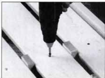
19 Position \frac{13}{16} -in.-wide spacer blocks between the slats, and screw the slats to the cross supports.
