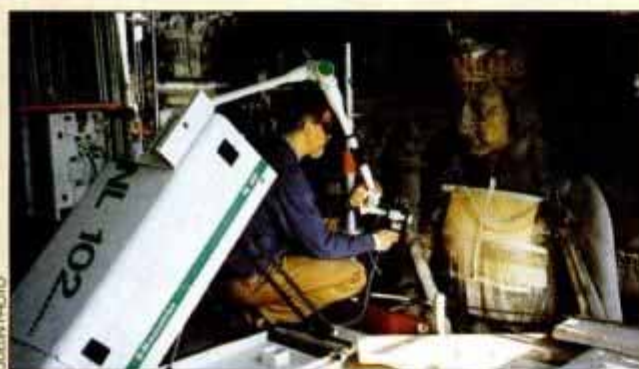
Artlight uses laser to loosen grime without abrading surface. The technique preserves weakened and polychromatic stone.
