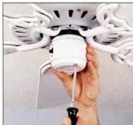
14 To install the light kit, remove the two screws that hold the bottom cap onto the switch housing and take off the cap.
