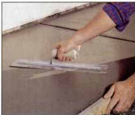
21 Hold the trowel flat and apply more pressure to its trailing edge to prevent it from chattering. Sweep it in wide arcs.
