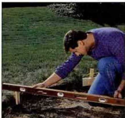
5 The first step in installing a curved form is to drive a grade stake. Use a level to check that the stake height is correct.
