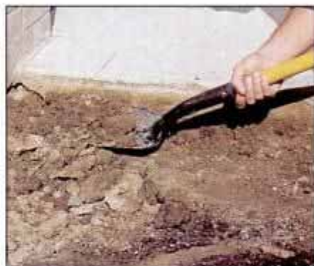
8 Use a pointed shovel—held at a shallow angle—to shave excess soil from the form bed. This prevents over-excavation.
