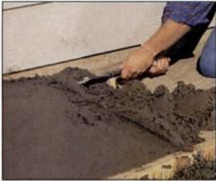
15 Every 5 to 6 ft., withdraw the screed pipe from the concrete. Leave the screed stakes buried in the slab.
