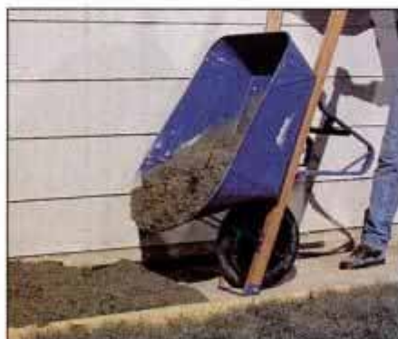
13 Use heavy-duty wheelbarrows to haul concrete to the forms. While one person hauls, another spreads the concrete.
