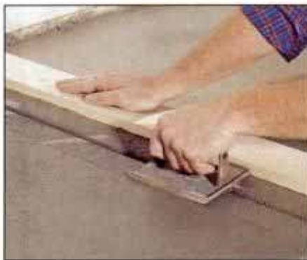
19 To make a control joint, lay a 1 x 4 down as a guide, then run a groover along it. Place a control joint every 40 in.
