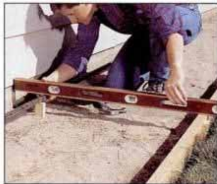
12 The screed pipe must be positioned above the opposite form to produce a slight slope. Check this with a level.
