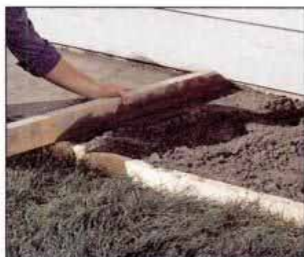
14 Once all the concrete is in the form, saw a screed board across the form. This strikes off excess concrete.
