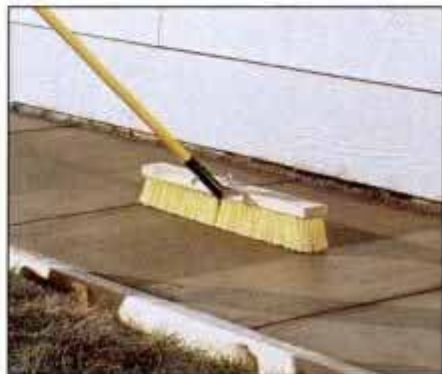
22 Use a broom to rough the surface for better traction. Cover the concrete with plastic for six days to keep it moist.
