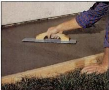
17 After all the concrete is poured, use a wooden or magnesium float to bring water and cement paste to the surface.
