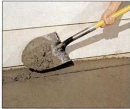
16 Use a shovel to sprinkle new concrete into the gap left by the screed pipe. Work this rough concrete smooth using a float.
