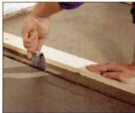
20 Cut into the control joint every few inches with a pointed trowel. This ensures that cracks will be under the joint.
