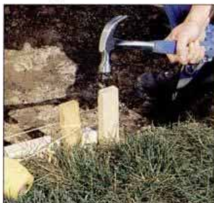
2 Drive 1 × 2 pine stakes next to the form lumber. Align the stakes using a string pulled taut between two stakes.
