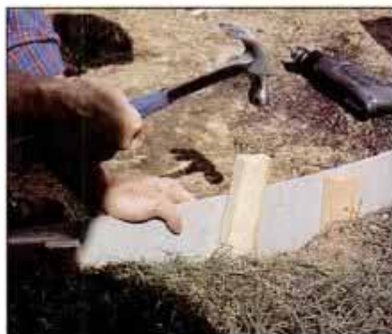
7 Support the curved form with stakes spaced 18 in. apart. The 2 x 4 form is supported every 24 in.
