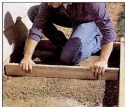
9 The form bed depth should be consistent. Use a 2 x 4 to drag the bottom of the bed until the same depth is achieved.
