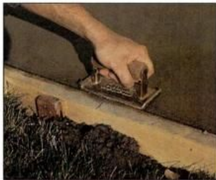
18 Use an edger to round the concrete perimeter. This looks nicer and is less likely to chip than a square edge.
