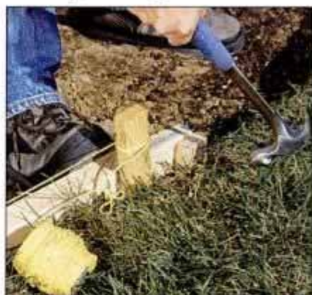
3 Drive a double-headed nail through each stake and into the form behind it. This kind of nail is easily removed.
