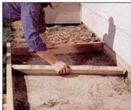
10 Put the finishing touch on the form bed by filling in the low spots with sand. Don't fill these spots with soil or concrete.
