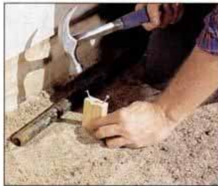
11 Drive screed stakes along the length of the form. Drive a pair of angled nails into each stake to hold the pipe in place.
