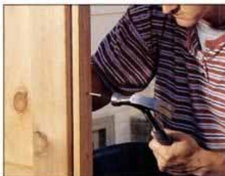
17 To withstand repeated closings, install a 1½-in.-wide × ¾-in.-thick gate stop on the post. Use galvanized nails or deck screws.
