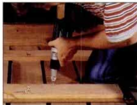
12 Lay out the gate slats and align the ends. Then, cut the crossmembers to length and secure them with screws.
