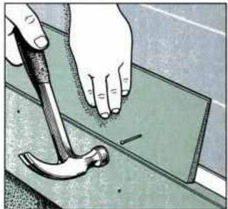
13 Nail the siding board in place—about 1 1/4 in. above the bottom of the board—to just clear the starter strip.
