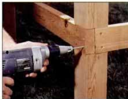
8 At the corners, you'll have two notches. Drive screws into the post and into the end of the adjoining rail.
