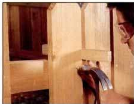
10 Align the slat tops with a string stretched from post to post. Space the slats with a \frac{3}{4} -in.-thick strip, and nail.
