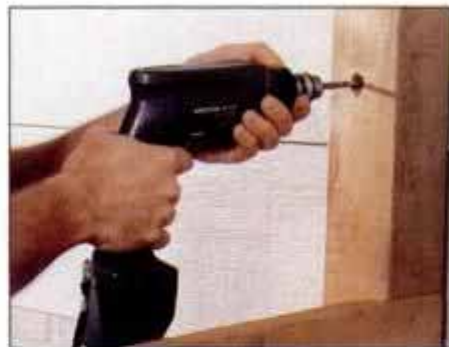
9 To secure a post to the house, first counterbore a \frac{1}{2} \times 1\frac{1}{2} -in.-deep hole. Then, drive a deck screw into the siding.
