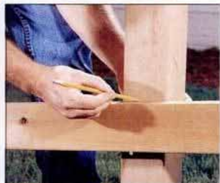
4 Position the uncut rails on the partially driven nails, and scribe the notch locations on the posts with a pencil.
