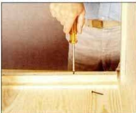
9 Install the ledgers to two opposite lower rails with screws and glue. Counter-sink pilot holes for flat head screws.
