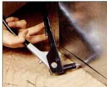
13 To assemble liner, first bore 1/8-in. holes, then install pop rivets. Use silicone caulk to make seams watertight.
