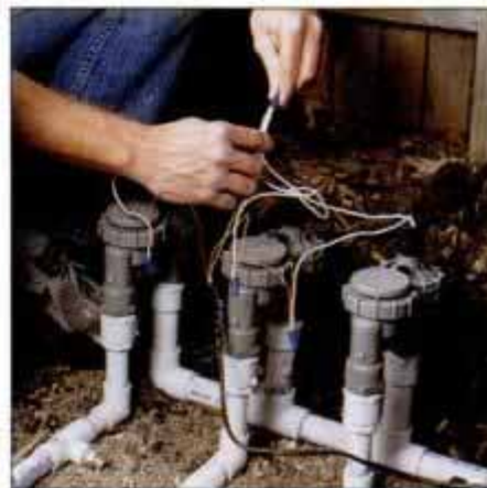
9 Attach white wire from control panel with the white wires from valves. Colored panel leads go to remaining valve leads.
