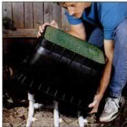
10 Cover the zone valve grouping with an access box and backfill the hole. The top of the box offers access to control valves.
