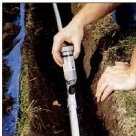
4 Dry-connect sprinkler heads to nipples and tees and compare height with grade. If necessary, try a longer or shorter nipple.
