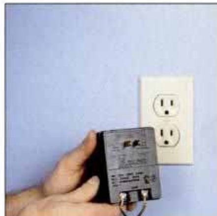
18 Finally, plug the transformer into the nearest power receptacle and program the control panel according to instructions.
