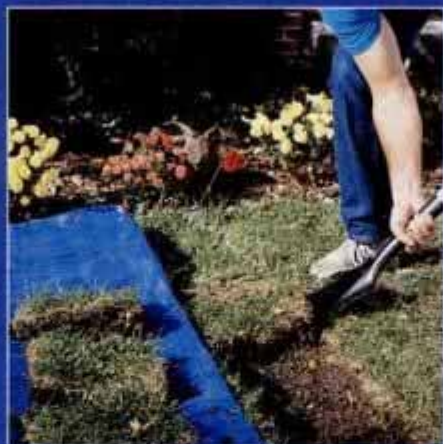
2 Begin the trenches by using a spade to slice out sod in squares. Set the sod on a tarp and dig the trenches 10 in. deep.
