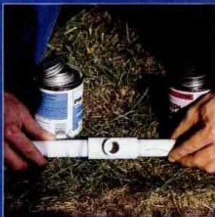
3 Splice tees into the sprinkler head supply pipes at head locations. Use joint primer and PVC cement to connect the tees.
