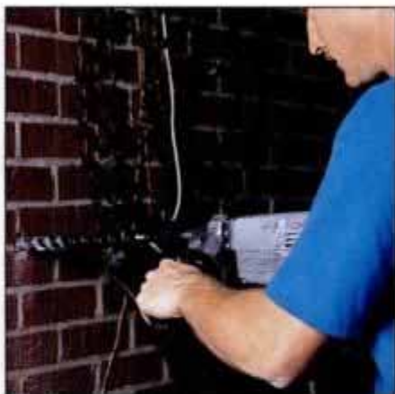
11 Bore a hole for pipe and low-voltage cable. If your home has a brick facade, start with a hammer drill and masonry bit.
