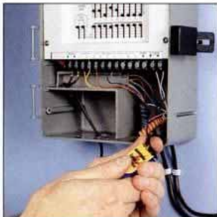
17 Attach a 9-volt battery to its harness inside the control panel. The battery saves the program during power outages.
