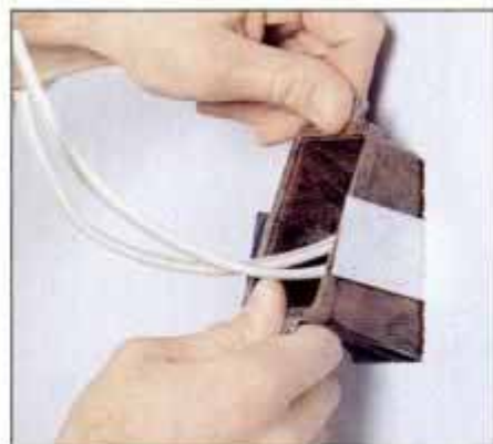
13 Pull the cables into the cut-in box and press the box into the wall. Then tighten the bracket screw securely.
