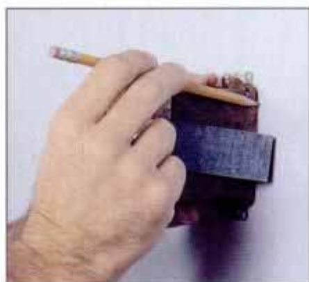
11 Determine the precise location of your switch box, then hold a cut-in box in this spot and trace around it.
