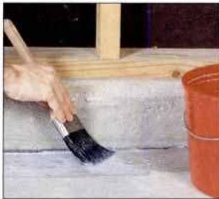
5 Begin applying the sealer by cutting in the entire perimeter of the floor. Be sure to use a stiff-bristle paintbrush.
