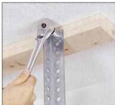
11 Attach a 2 x 4 cleat to the ceiling where the joists fall. Then lag a piece of angle-iron to the side of the cleat.
