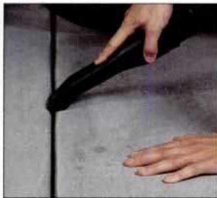
2 Be sure to vacuum any loose debris from control joints. Any material left behind will be trapped permanently.
