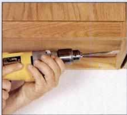
2 If necessary, bore a hole through the side partitions of adjoining cabinets so the fixtures can be joined with conduit.
