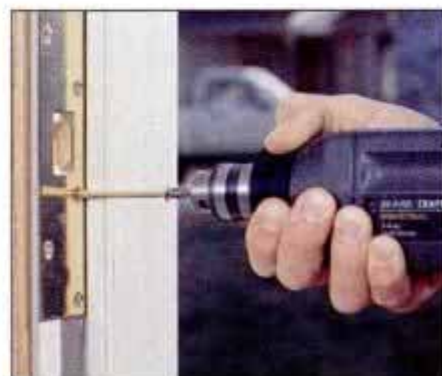
12 After testing the operation of the lock, secure the jamb plate by driving long screws into the jack studs.
