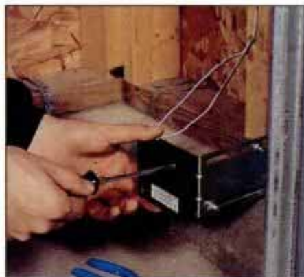
15 Install the L-brackets on the jack studs for the door opening. Then attach the infrared sensors to the brackets.
