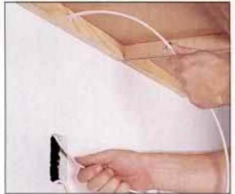
8 To run the cable between the fixture and the switch, feed the cable through the cabinet hole, down to the opening.
