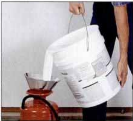
4 Pour sealant into a paint bucket for cutting-in purposes, then fill a low-pressure sprayer for the larger areas.
