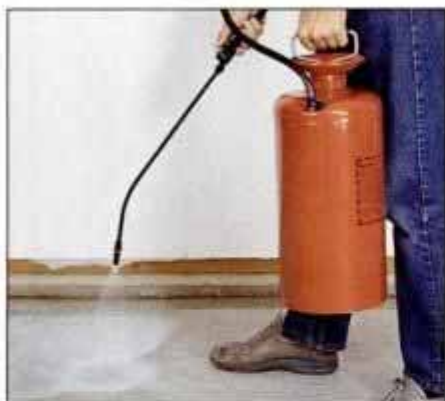
7 Using a standard garden sprayer, start in one corner of the floor and begin applying sealant in manageable segments.
