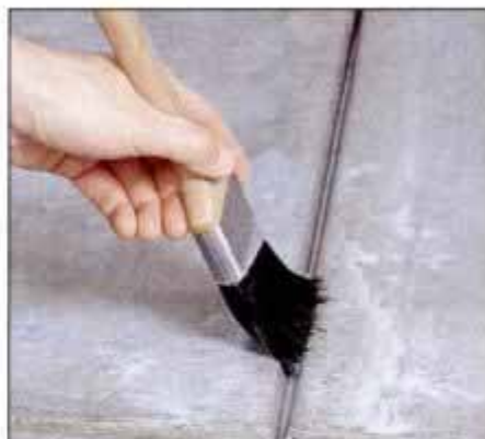
9 Any excess puddling of sealant in control joints or other depressions should be swept away with a brush.
