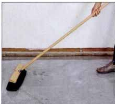
8 After allowing the sealant to penetrate for about 5 minutes, use a push broom to even out the coverage.
