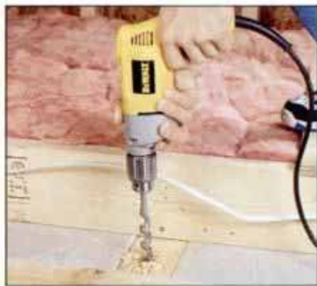
3 Determine the wall location of your new switch, then bore through the top plates of the same wall from above.
