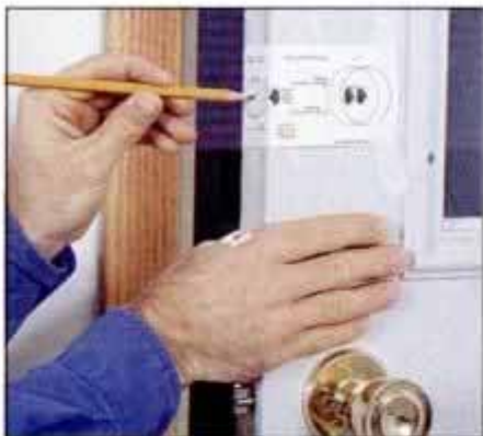
1 Locate the hole template on the edge of the door between 6 and 8 in. above the lockset. Mark the hole locations.
