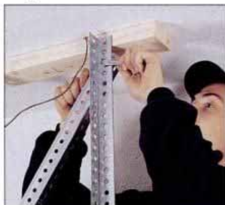
12 To control side-to-side movement, bolt a third piece of angle-iron diagonally between the two vertical hangers.
