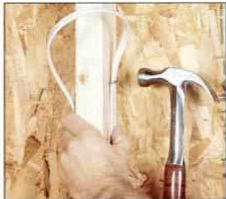
6 Bring cable up the attic or the gable wall that will support the floodlight and staple it alongside a convenient stud.
