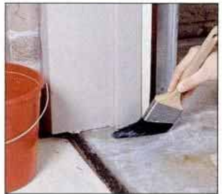
6 Take extra pains to apply sealer around areas that are open to the weather, like this garage door opening.
