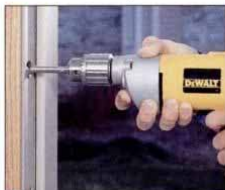
11 Locate the centerpoint of the pencil marks left on the jamb. Then bore the jamb hole to the proper depth.
