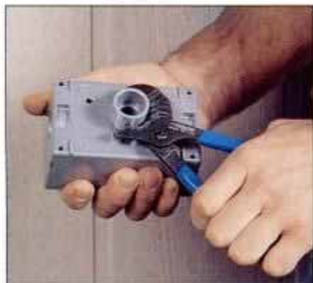
7 Turn a nipple or threaded adapter into the back of the box and feed the new cable through this extension.
