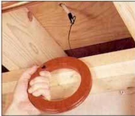
6 Using the fish tape, gently pull the cable into the basement. Avoid cutting or abrading the cable insulation.
