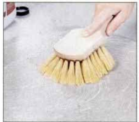
3 Use a stiff brush and a strong degreaser or concrete cleaner to remove oil spots and tire grime from the surface.
