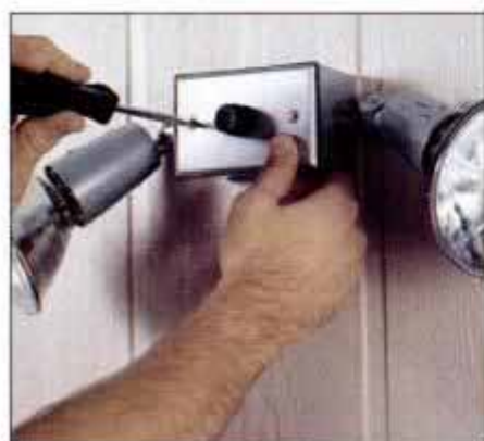
10 Push the sensor into the box, then press the fixture's rubber weather gasket in place. Tighten the cover securely.
