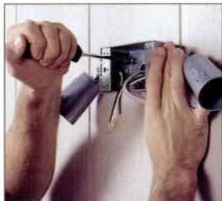
8 After installing a lamp holder on each end of the box, mount the box on the outside wall with two wood screws.
