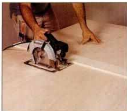
1 Cut the plywood panels to size using a circular saw. Clamp a guide to the panel and run the saw along it.
