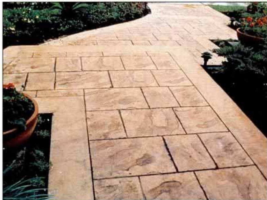
This walk is textured and colored to look like dry-laid red flagstone. The pattern choice in this paving system is unlimited. The stones can be all the same size, interlocked shapes, laid in rows or completely random in shape and pattern.
