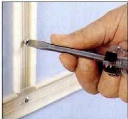
5 Secure the channel with drywall anchors and screws. At a T connection, break away the edge to make room for the wires.
