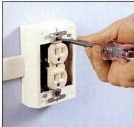
13 Finally, install the receptacles in the extension boxes just as you would in an ordinary in-wall receptacle box.
