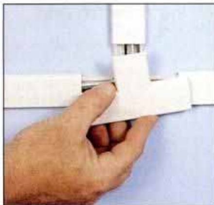
9 Snap connectors over the trim channels at T and L branches. Trim channels extend under connectors about \frac{1}{4} in.
