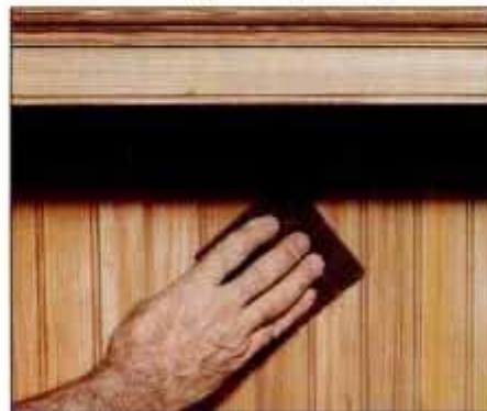
7 Clean small beading on tongue-and-groove back panels with stripper-dampened abrasive pad and small scrapers.
