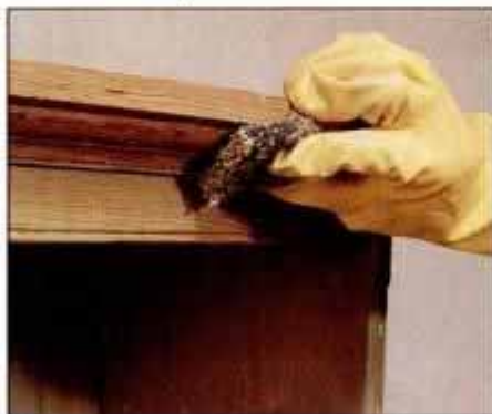
6 Where a large flat scraper can't reach, use a synthetic abrasive pad. Avoid steel wool with water-base products.
