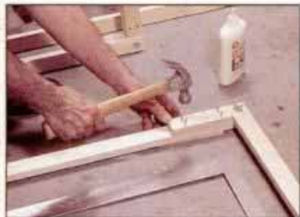
After cutting 1 x 2 stock to length, secure cleats to the ends of each long member. Set cleats back 1 1/2 in. from ends.
