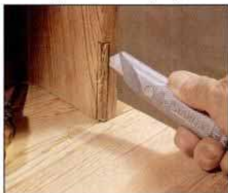
9 To repair this worn area on the case side, first use a sharp utility knife to define a uniform area to be cut away.
