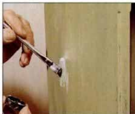
2 If you're unsure of the old finish, spot test with several strippers to determine the best. We used a water-base stripper.
