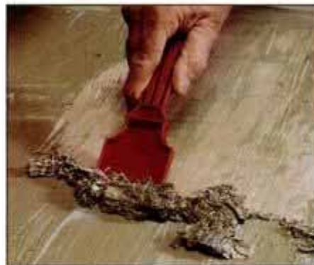
5 Use a scraper to remove the softened paint. Although gloves aren't required for a water-base stripper, they're a good idea.
