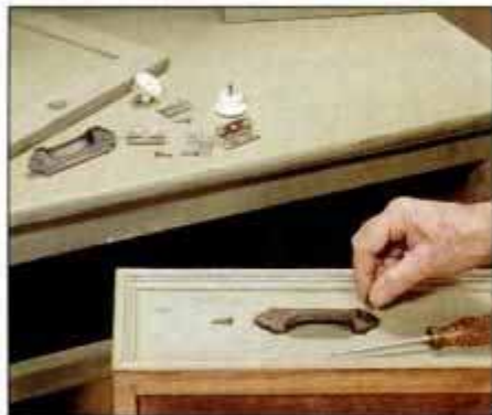
1 Begin the job by removing all hardware, doors and drawers. Check the condition of the hardware screw pilot holes.
