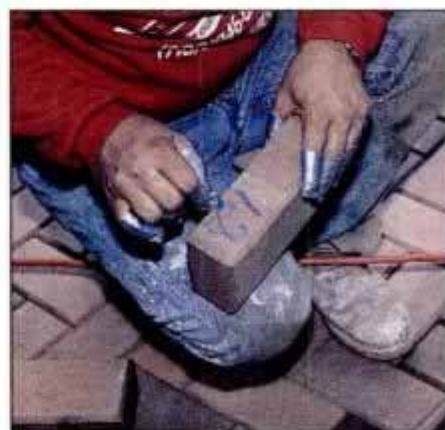
15 Pick up each brick from the pattern that needs cutting and number it in sequence so it can be replaced easily later.
