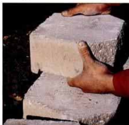
9 As you stack the blocks, make sure to fully engage the retaining lip on the back of each with the course below.
