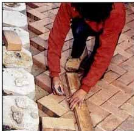
14 When the pattern reaches the other side of the drive, stretch a string for the shoulder course and mark the bricks.
