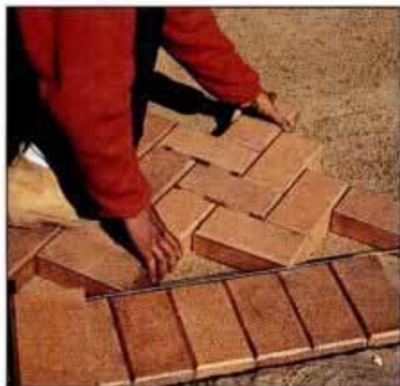
13 Set the bricks for the shoulder course on one side of the drive, and then start with the overall pattern in one corner.
