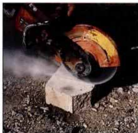
8 Measure, mark and cut the blocks to size with a masonry saw or with a masonry blade installed in a circular saw.
