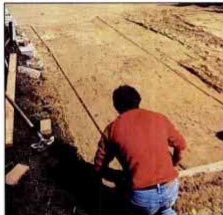
12 Using a 2 × 6 board that spans the width of the bars, screed the sand base to a uniform height. Fill any gaps as you go.
