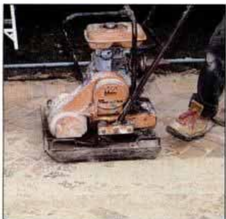
19 With all the pavers in place, spread a thin layer of sand over the surface and force it into the cracks with the vibrator.
