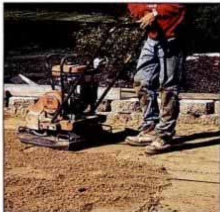
10 Spread out the sand for the setting bed, and then compact it with a rented vibrator to a depth of about 1½ in.
