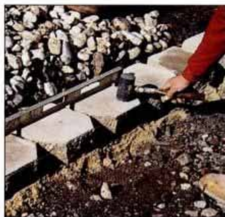
6 Spread a base of fine sand where the retaining wall will be, and then start installing the block. Level each in place.
