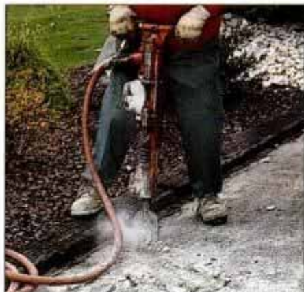
1 Begin by breaking up old asphalt or concrete. Use an air hammer and a compressor or work with a pick and prybar.
