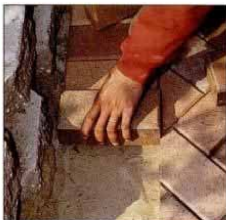
18 Once all the cut pieces are in place, install the shoulder course, making sure each brick is flush.
