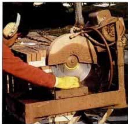
16 Cut the bricks with a rented, water-cooled masonry saw. Cut each paver \frac{1}{4} in. shorter than the mark.
