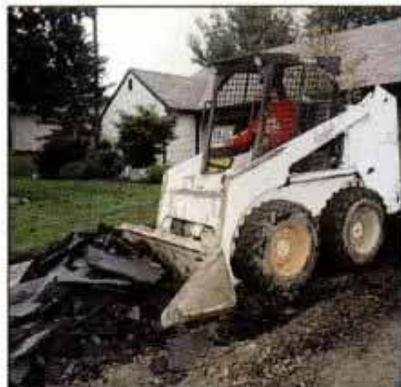
2 Remove all the concrete or asphalt debris. Then excavate to the proper depth to accommodate the subbase and the pavers.
