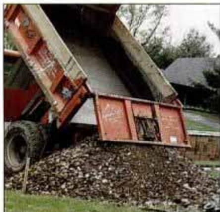
4 Then install the secondary subbase by spreading a blended layer of crushed concrete and \frac{3}{4} -in. crushed stone.
