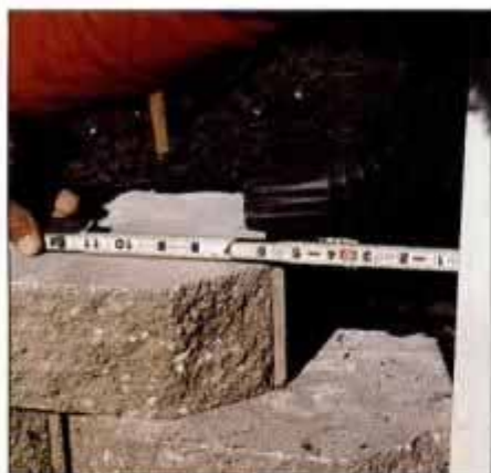
7 Stagger the courses of block as you go up. It's better to align the full blocks first, and then cut the half blocks to fit.
