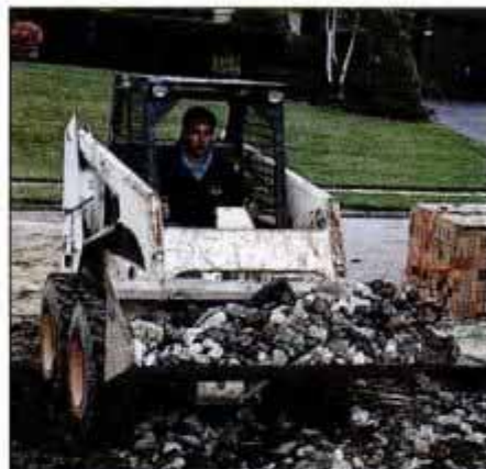
3 Once the surface is prepared, lay down a 6-in.-thick layer of reprocessed concrete to establish the primary subbase.
