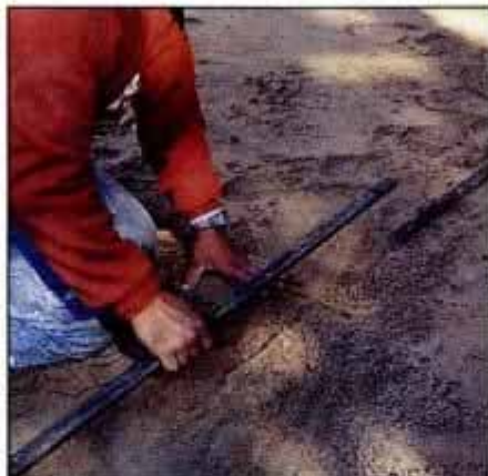
11 Embed flat steel screeding bars in the sand bed. Adjust the height of the bars to match the bottom surface of the pavers.
