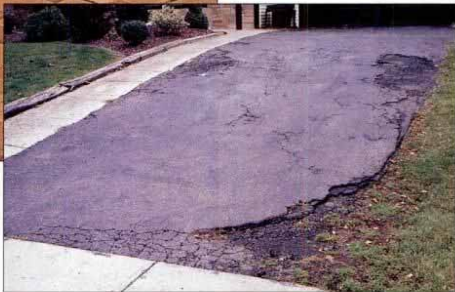
This badly cracked and broken asphalt driveway was a perfect candidate for replacement. Brick pavers are a very durable and attractive alternative to asphalt and concrete.
