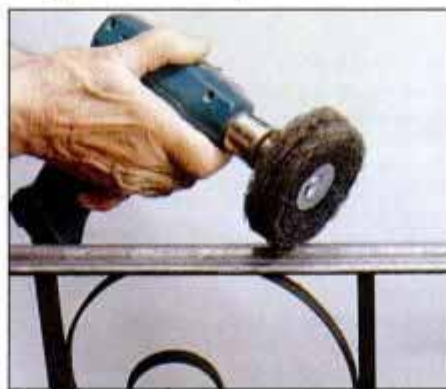
8 Clean off remaining rust with an abrasive wheel. We used the 3M Paint and Rust Stripper with good results.
