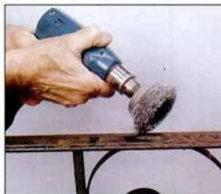
7 Remove large pieces of loosened paint and loose rust using a wire wheel chucked into an electric drill.
